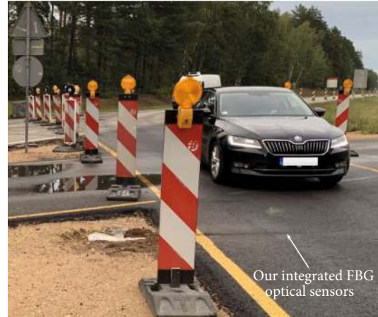
FIGURE 3: Embedded FBG sensors on the carriageway in the location (b).
