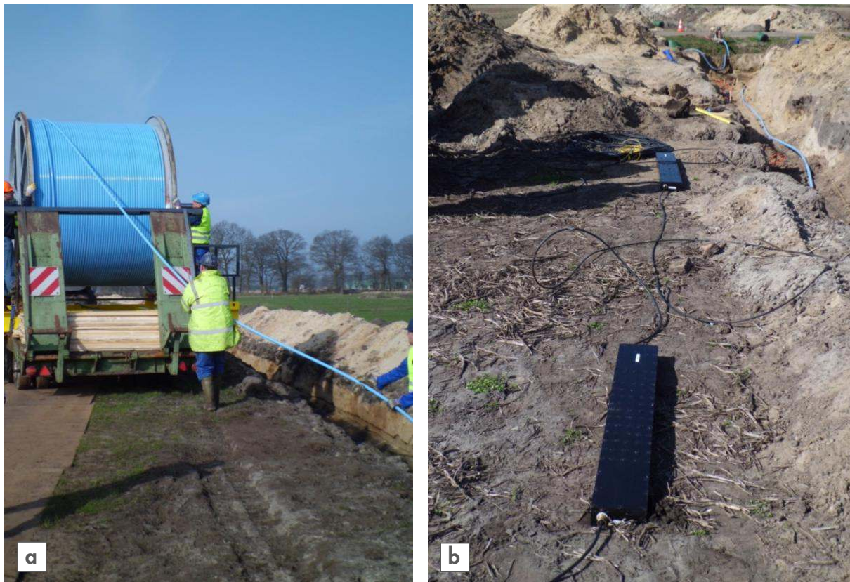
Figure 8.9: Deployment of prototype cables in Schoonebeek for a surface seismic field trial. (a) Broadside-sensitive cable is spooled from a transport reel and positioned in a trench. (b) Several component-selective prototype sensors installed in a ruggedized box, ready for deployment next to the broadside-sensitive cable prototype in the trench. [97]
