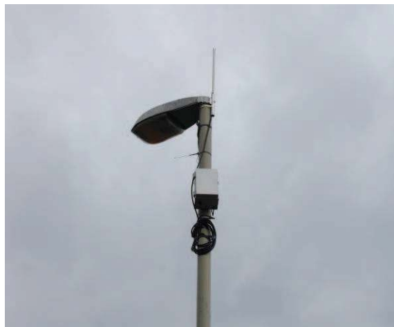
Figure 3- Autonomous Zigbee-GPRS gateway mounted on a lamp column in Leicester
