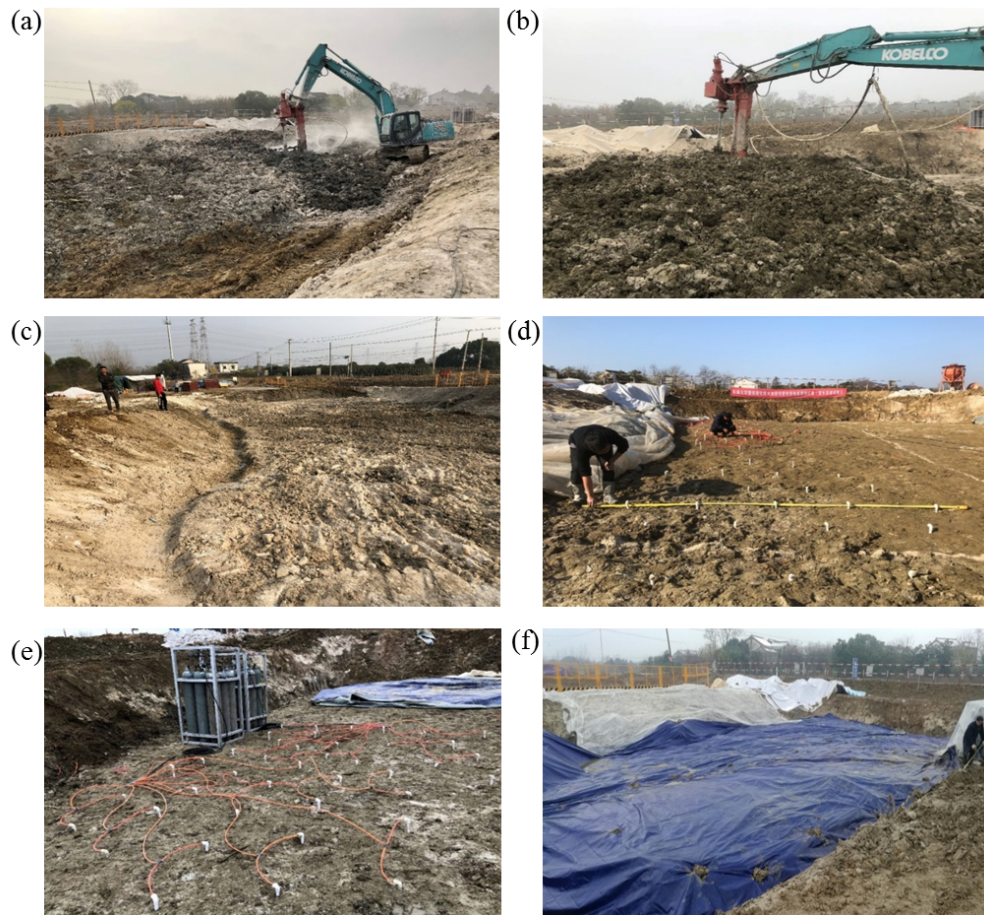
Fig. 5. Overview of in-situ construction procedure for mass carbonation treatment: (a) mixing MgO powder; (b) secondary mixing; (c) ditching; (d) inserting PVC; (e) connecting vent pipe; and (f) sealing and carbonating.
