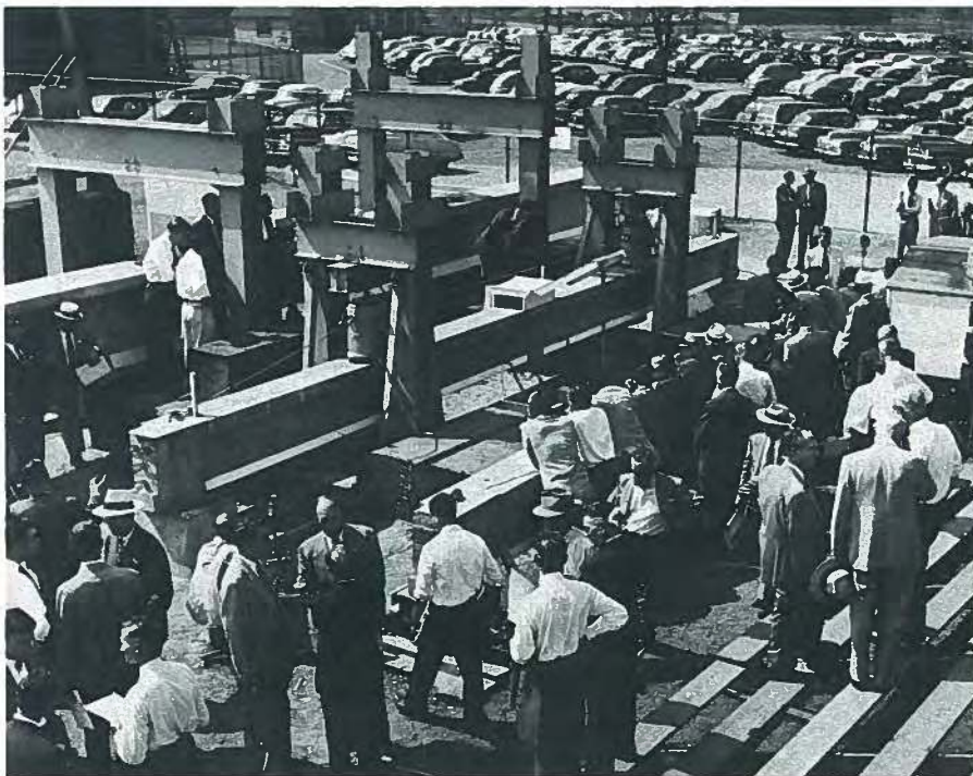
Fig. 37. An overflow crowd of invited guests witnessed the Austin Company tests in 1951. Three full-scale girders [two 40-ft (12.2 m) and one 60-ft (18.3) girders] were load tested using hydraulic jacks.
