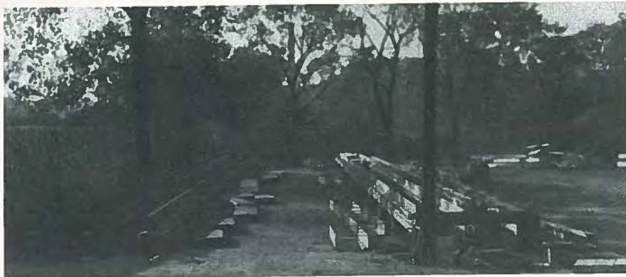
Fig. 16. Fabricating beds at a Breeko plant for producing pretensioned channel slabs with deflected strands. Built in March 1953.
