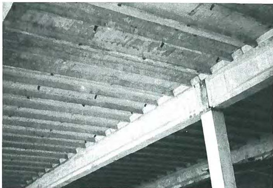
Fig. 10. A 6-ft (1.83 m) wide double-tee was developed from existing channel slab designs to allow larger spans between beams in the cold storage warehouse for Beatrice Foods.
