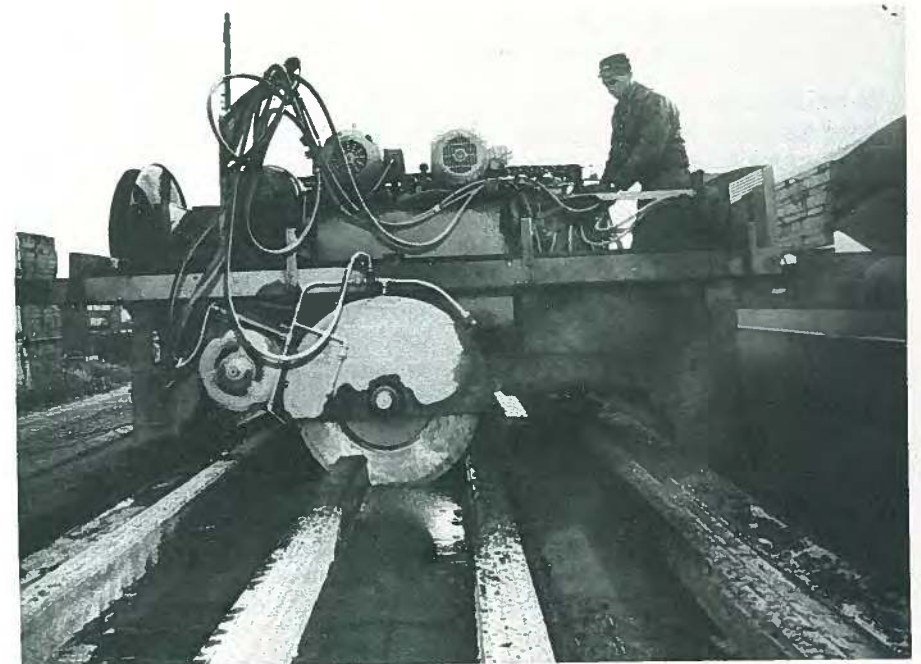
Fig. 26. After the concrete set, the Quadeck was cut to size by a saw attached to the machine.
