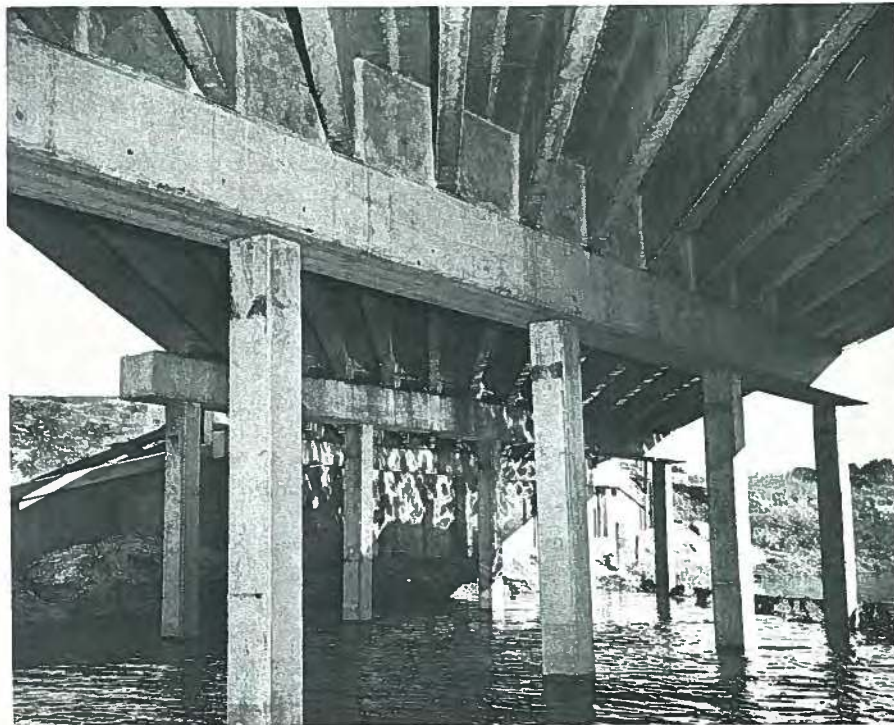
Fig. 16. Underside of precast prestressed county bridge in Sarasota, Florida. Courtesy: Paul Zia.
