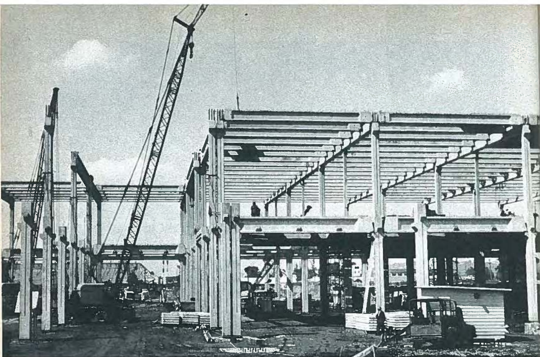
Fig. 42. Erection of giant Boeing Company development center in Seattle, Washington, 1956. The two-story 400 x 600 ft (122 x 183 m) precast prestressed structure with 40 x 60 ft (12.2 x 18.3 m) bays was completed in 7 months and at the time was the largest industrial-type prestressed building in the world.
