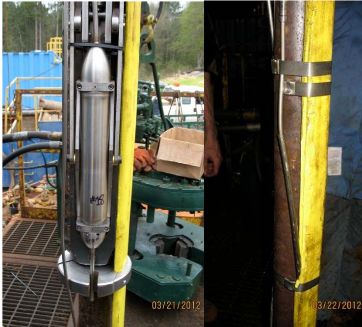
Figure 4 (left) MBM Geophone with hydraulic clamp, mounted on tubing with yellow flatpack. (right) Flatpack with hydraulic line, each attached to tubing with steel banding. The DAS data was recorded using a fiber inside the flatpack, clamped to tubing as shown with clamps every ~10 m and banding every ~5 m.
