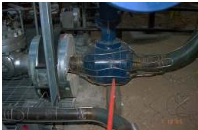
Figure Q-4. Valves can be kept warm overnight, independently of the surrounding pipe, if a separate heat trace circuit is applied to the valve. This reduces parasitics because the pipe heaters can be turned off at night. In this photo, the same heat trace circuit was applied to the valve and surrounding pipe. During the rework of the heat trace system in 1996, separate valve circuits were installed on valves 4 inches in diameter and bigger.
