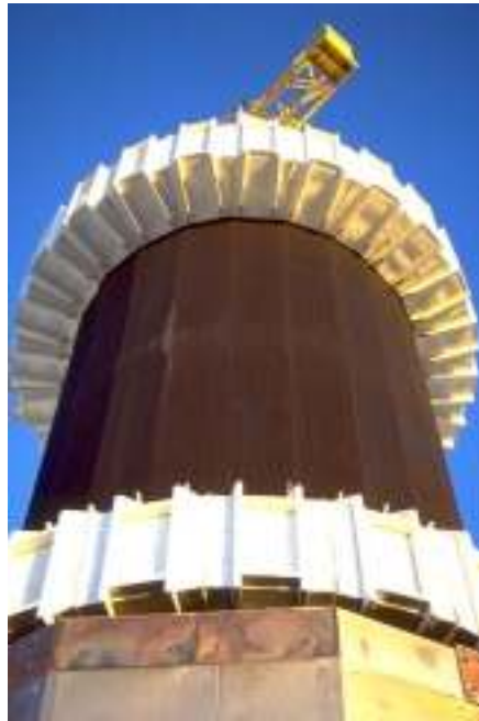
Figure 3-1. Close-up of Solar Two receiver.
