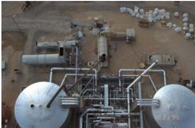
Figure L-5. Overhead view of the salt fill operation; the hot tank is on the left and the cold tank is on the right.
