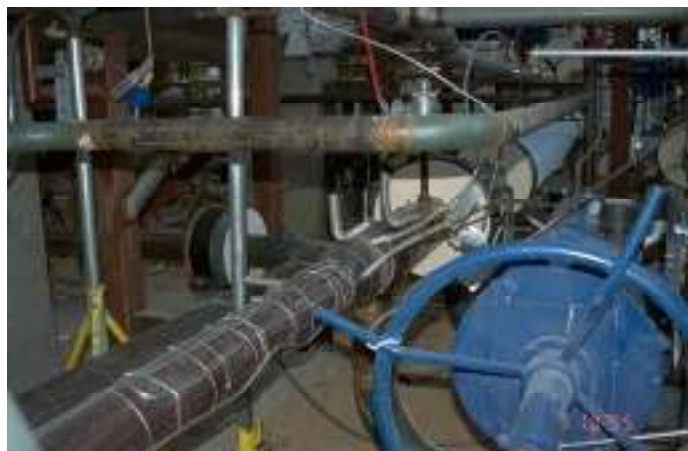
Figure Q-3. Multiple heat trace cables were applied to pipes that drained nightly to allow a two-hour heatup time the next morning. One or two spare cables were installed as well. A lesson learned was that heat trace must be installed uniformly (i.e. constant value of W/ft); otherwise, hot spots can occur that lead to pipe corrosion. A nonuniform section of heat trace is seen in this photo (see loop back). During the rework of the heat trace system in 1996, nonuniformities were eliminated.
