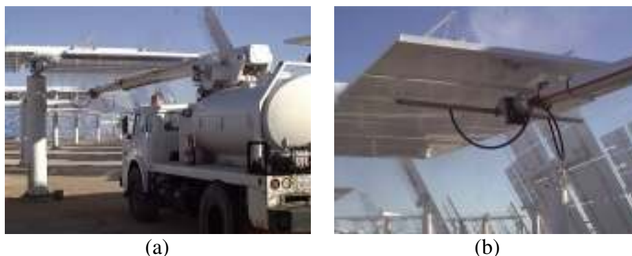
Figure 2-6. The Solar Two wash truck (a) and close-up of spray bar (b).
