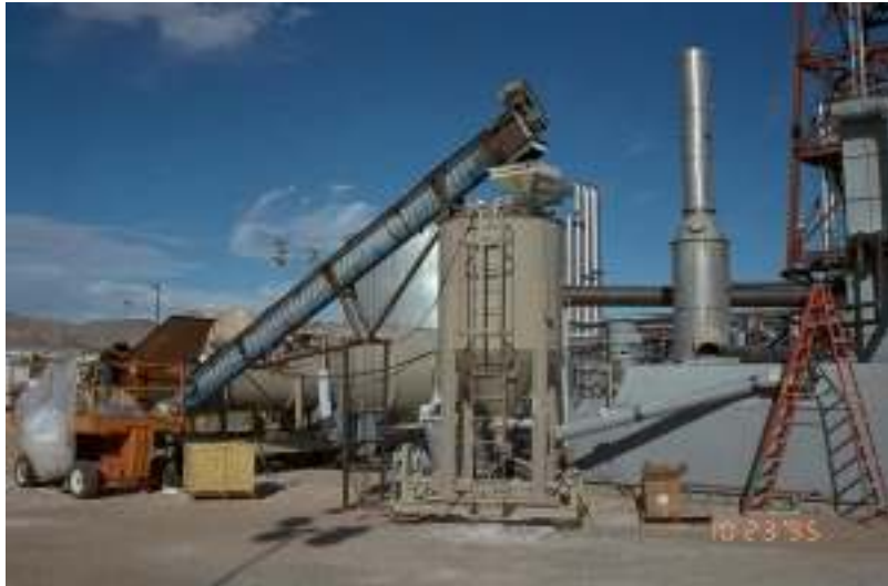
Figure 4-4. Conveyor belt feeding crushed salt from the hammer mill into the salt hopper. The screw auger can be seen as the pipe feeding into the wall next to the ladder.
