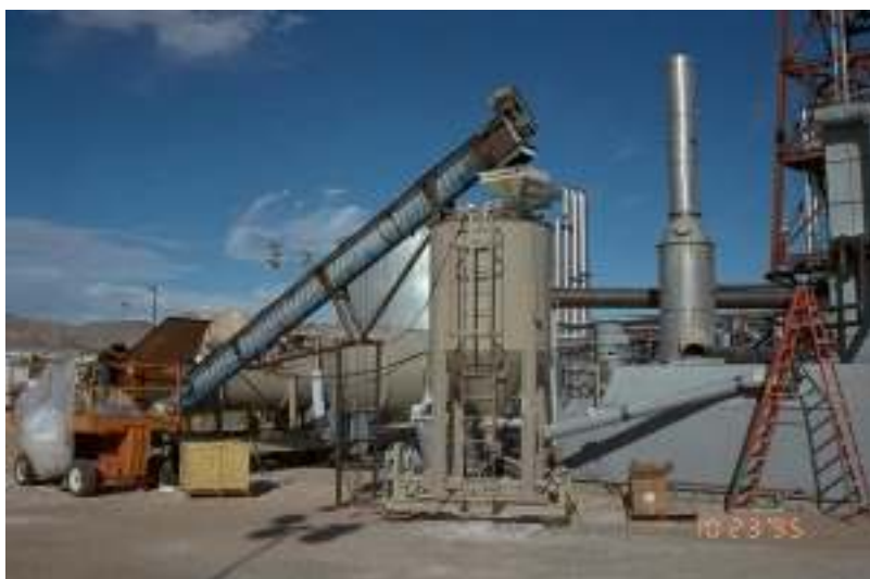
Figure L-4. Conveyor belt feeding crushed salt from the hammer mill into the salt hopper. The screw auger can be seen as the pipe feeding into the wall next to the ladder. The vent stack to dilute the NO x can be seen in the background.
