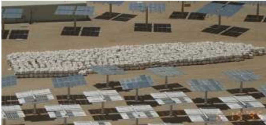
Figure L-1. 1.3 million kg (2.8 million pounds) of nitrate salt awaiting melting at Solar Two.
