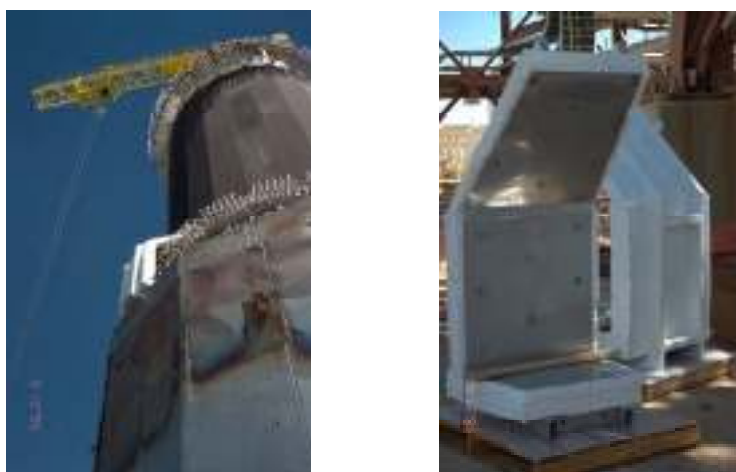
Figure Q-2. Ovens structures surround the receiver header pipes. Seals must be good for ovens to be effective. Sealing problems often made it difficult to heat up the ovens on the windward side of the receiver.
