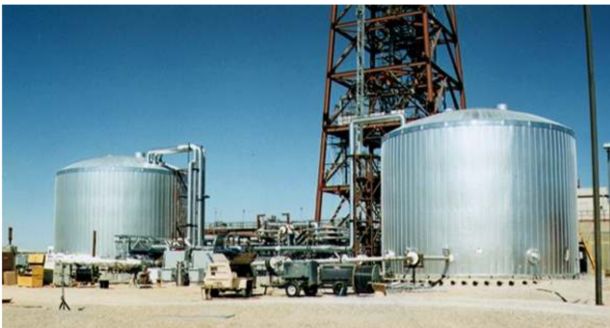
Figure 4-1. Cold (left) and hot (right) nitrate salt storage tanks.
