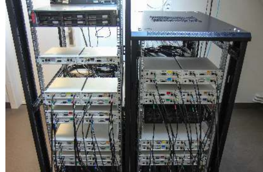
Fig. 8: Measurement setup: Power gain variations across the array were calculated from LTE-like uplink data symbols in the KUL massive MIMO testbed. 32 antennas were used in this measurement.
