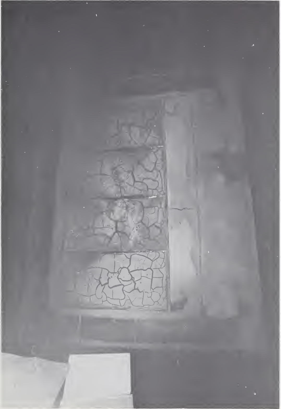
Figure 17. The fire side of the wall panel after it was removed from the surface just before extinguishment of the fire.
