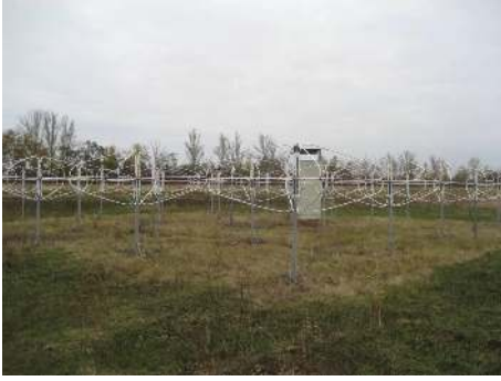
FIGURE 1: Active antenna array of 5 \times 5 elements as a basic part of the GURT radio telescope.
