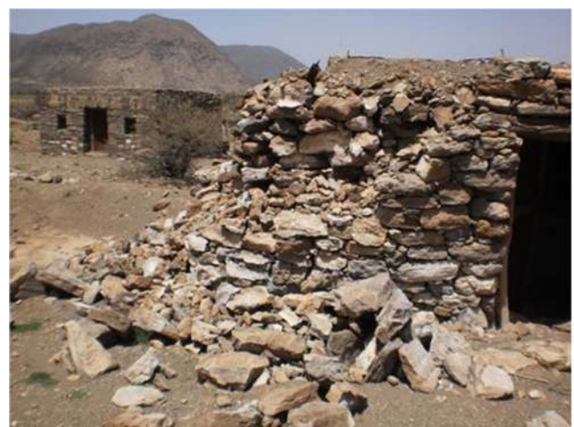
Fig. 5 Building damaged by the 31 March 2011 earthquake. Better constructed walls, as seen in the background, sustained only cracking
