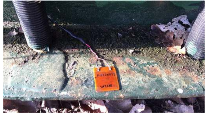
Fig. 12. Attached FSM transducer on the 4 m diameter tank floor without any surface preparation.
