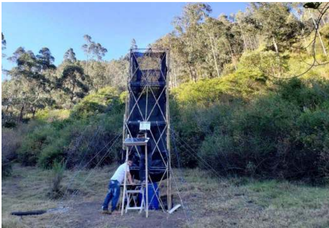
Fig. 9 Installation of sensors fog collector system
