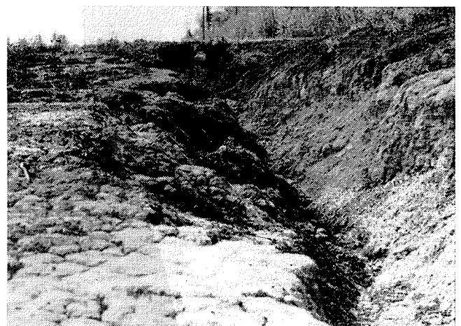
Figure 4. Poor road construction is evidenced by this actively eroding side ditch which will continue to be a source of both undesirable sediment and excessive maintenance for many years.
