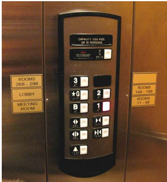
Fig. 6.13 An elevator that has both good and bad SR features. The open button is closer to the doors (which are to the left , not shown), but the rooms do not map easily to the buttons, 100-level rooms are on floor 2, which does not match many of the most direct mental models, such as 100-numbered rooms being on floor 1, or floor 3 being above 2
