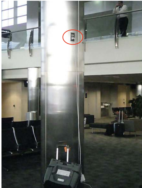
Fig. 12.3 An electrical outlet ( circled ) on a column designed to be difficult to use?
