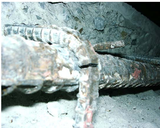
Fig. 3 Example of fractured steel bar.
