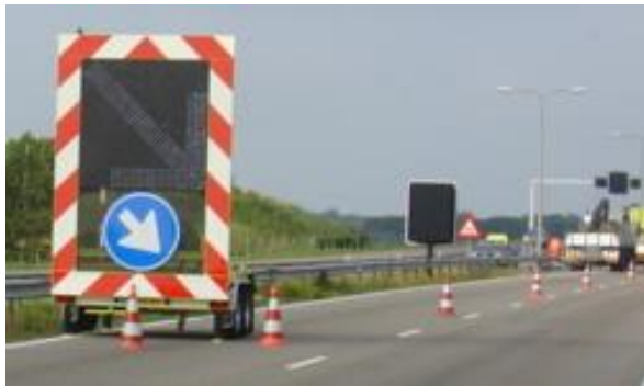
Figure 2.3: Traffic cones as channelizing device.
