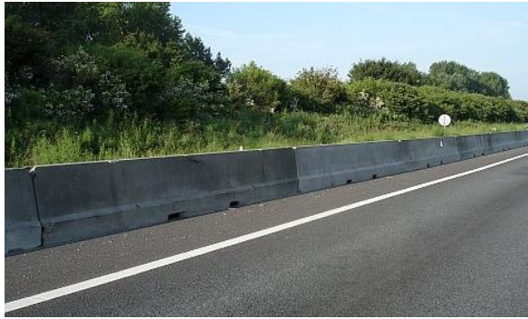
Figure 2.1: Concrete barrier as channelizing device.
