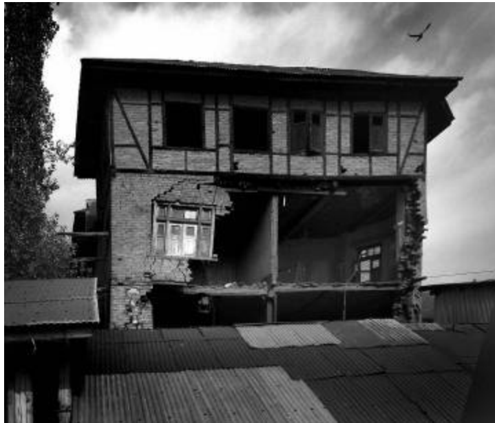
Figure 3: House in Baramula, Kashmir damaged in 2005 earthquake showing how unreinforced masonry collapsed, leaving the top story of Dhajji Dewari in place.
