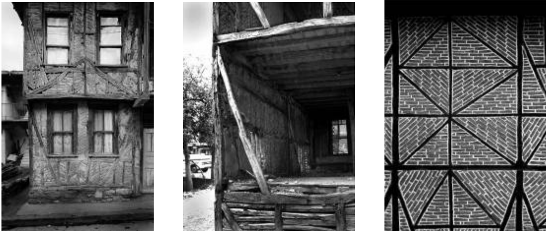
Figure 7: (a) Himis house in Gölcük damage district after the 1999 earthquake with no visible damage.
