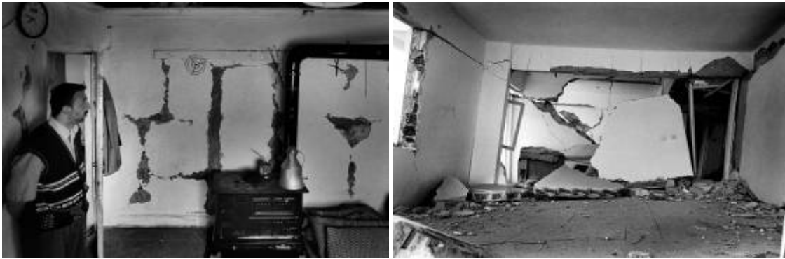
Figure 16: (a) Interior of house in Orta, 2000, showing the working of the himis wall construction. (b) Ruptured frame and collapsed masonry infill in Gölçük RC building after 1999 earthquake.
