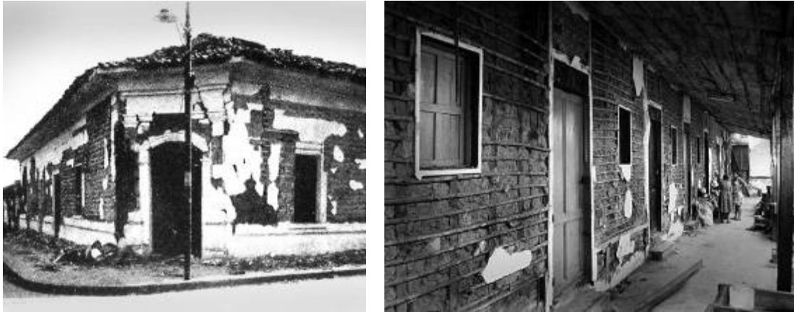
Figure 11: (a) J.R. Freeman's photo of Taquezal building in Managua after 1931 earthquake. (b) San Salvador Bahareque building after 1986 earthquake showing a similar plaster shedding.
