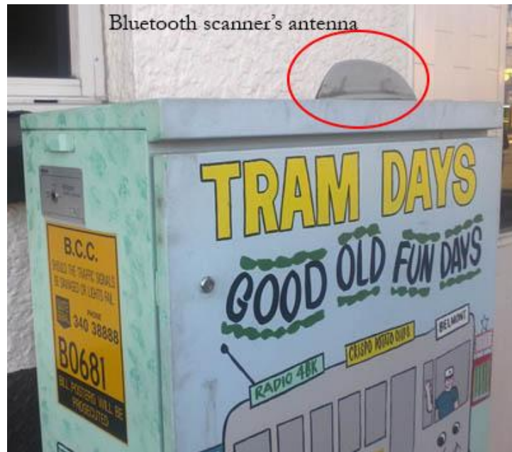
Figure 7: A photograph of a BMS equipped signal controlled in Brisbane with a shark fin shaped BMS antenna on the top
