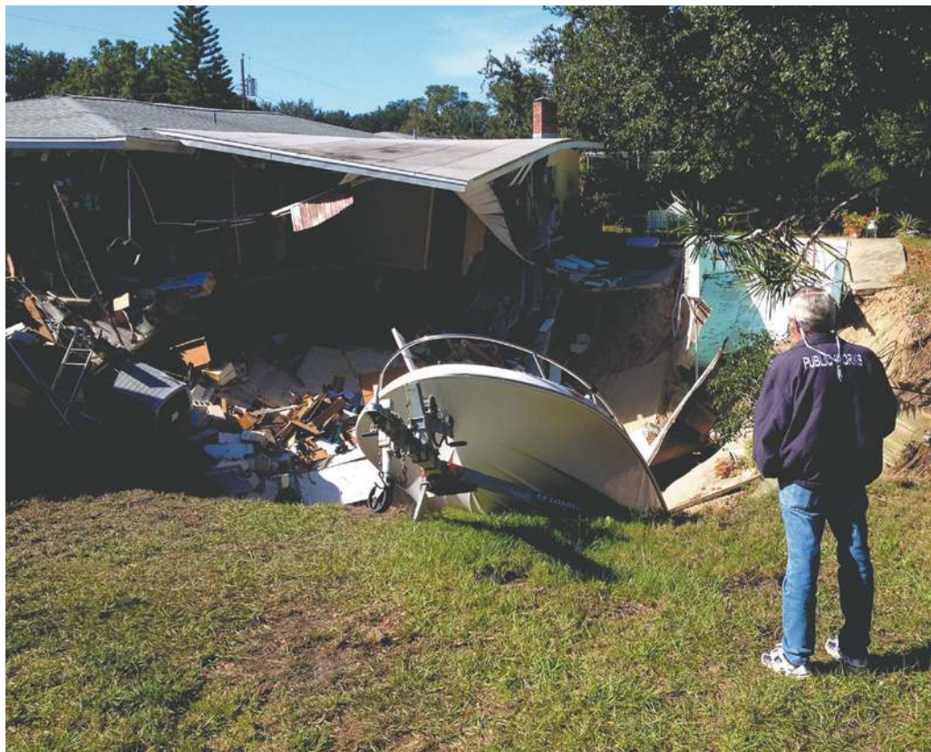
Grounds for concern: a sinkhole in Florida devoured a pool, a boat and two houses on 14 November.
