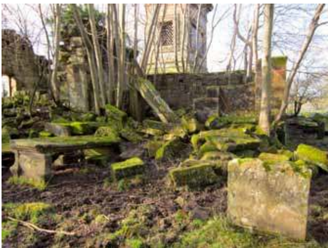
Figure 96: View showing the poor condition of the landscape at St Michael's Churchyard, Cambusnethan, North Lanarkshire. The graveyard, along with three mausolea, is Category B listed. The graveyard contains several late-medieval grave-slabs and an early medieval cross-shaft was discovered here in 1898. © Susan Buckham
