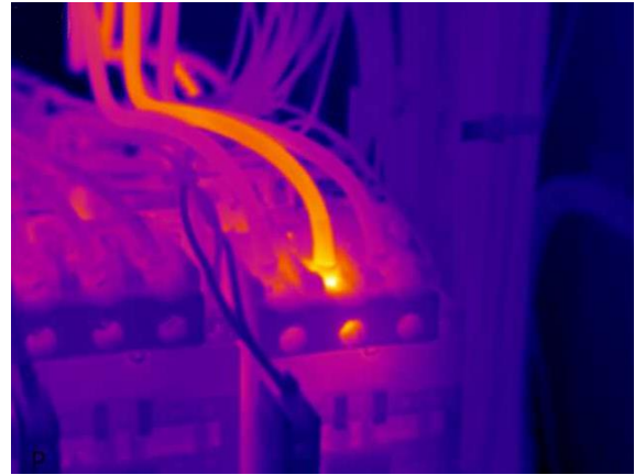
Fig.8. Examples of defects which can be determined during the thermal imaging diagnostics. Exceeding a permissible temperature of a conductor for one phase (a thermogram).
