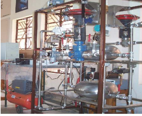
FIGURE 1: Photograph of the pneumatic pressure system.
