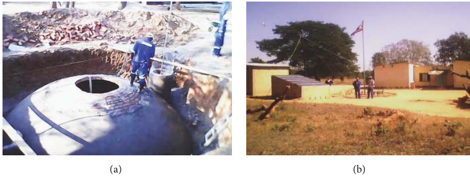
FIGURE 1: (a) 50 m 3 biogas digester under construction and (b) rural administrative office solar panels and photovoltaic power line shown next to the single standing individual [11, 14].
