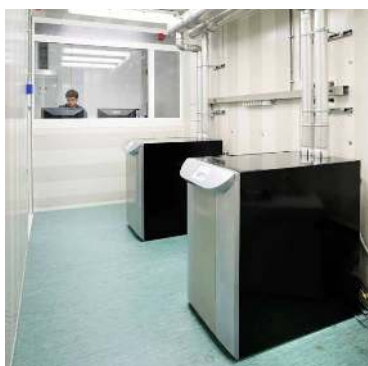
Figure 18.13: Mk5-based CHP system prototypes in the MTT test cell.
