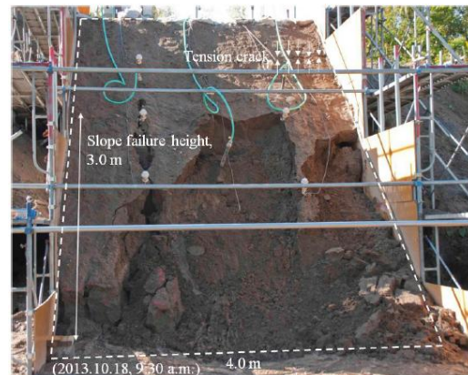
Fig. 16. Slope failure observed at October 17, 2013.
