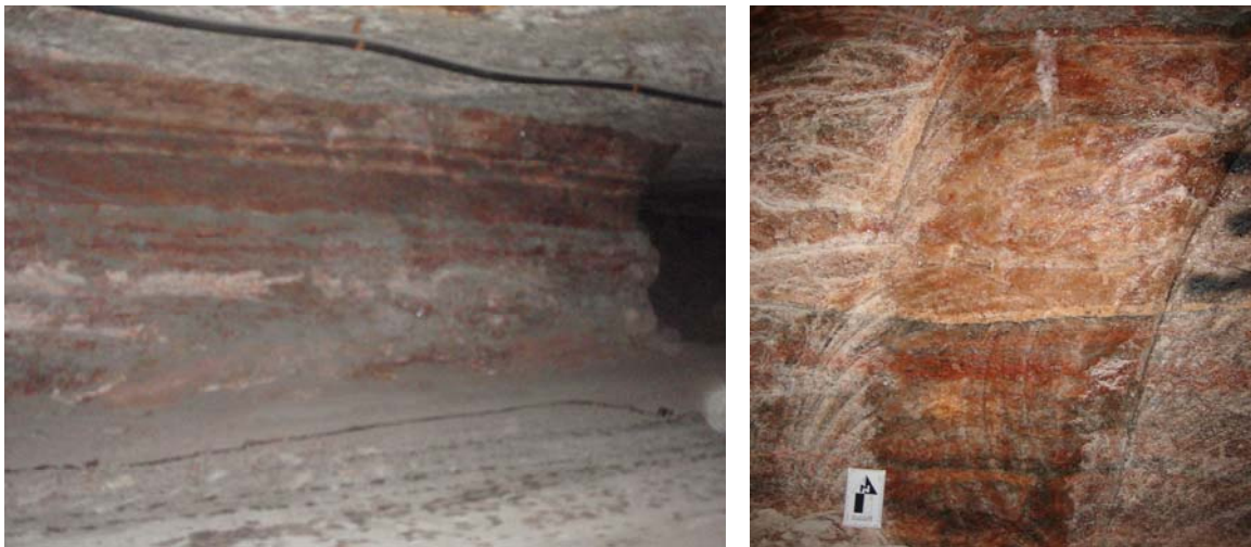
Pictures of clay strings and bedding planes in Mosaic Mine (pillar and close-up)
