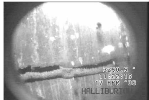
Images of Joint 82 Casing Damage at a Depth of 3,250 Feet.
