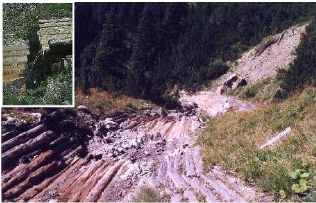
Fig. 2. The wooden drainage system is disrupted by the eroding power of debris flows, by small slides from the adjacent slopes (top right) and by differential movements within the landslide (detail top left), which leads to increased displacements rates.
