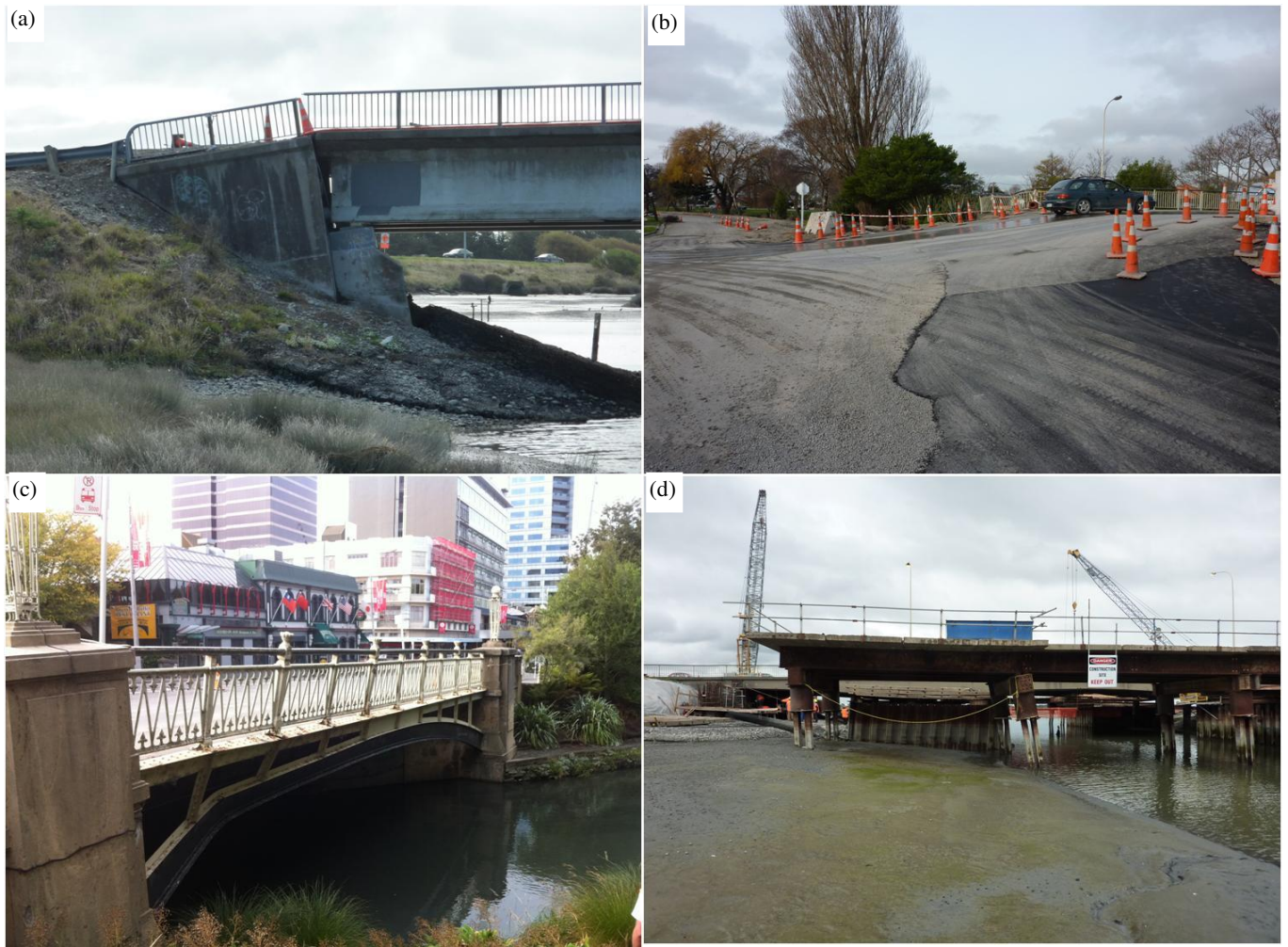
Figure 26: Summary of bridge damage: (a) back-rotation and settlement of the western abutment of South Brighton bridge; (b) settlement of the northern approach of Gayhurst Road bridge following the June 13 2011 earthquake; (c) abutment back-rotation and buckling of the steel arches of Colombo Street bridge; and (d) movement of temporary construction platform for Ferrymead bridge due to lateral spreading.
