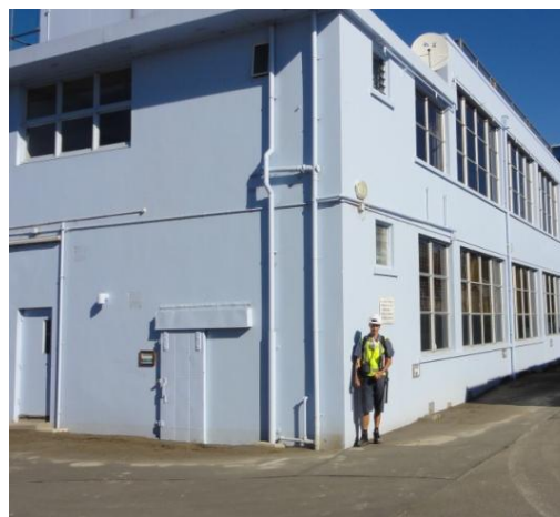
Figure 12: Two-storey building that underwent liquefaction-induced punching movements [7].
