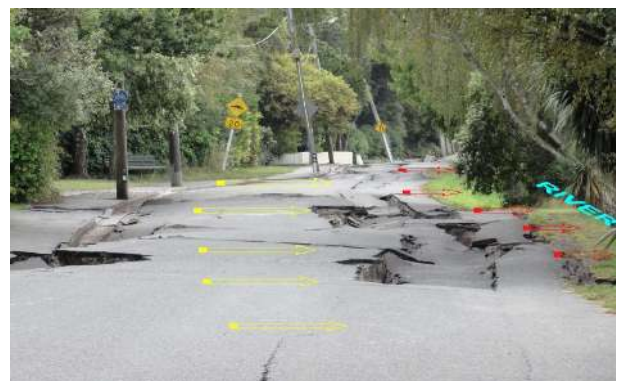
Figure 24: Lateral spreading toward the Avon River.
