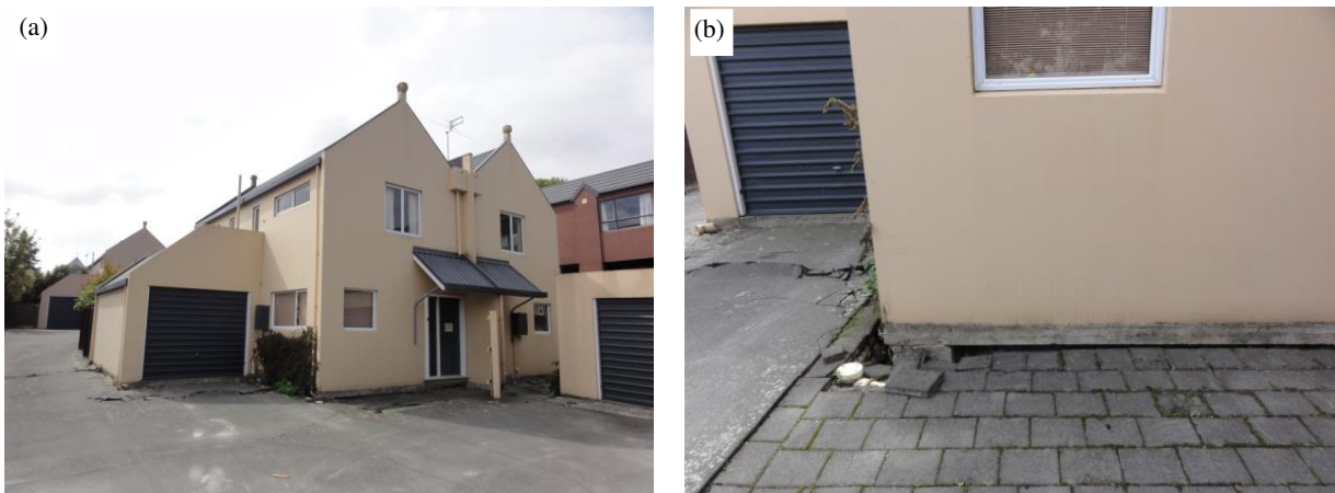
Figure 11: Duplex housing complex: (a) looking north at centre building, and (b) close-up of ground settlement next to centre building [7].
