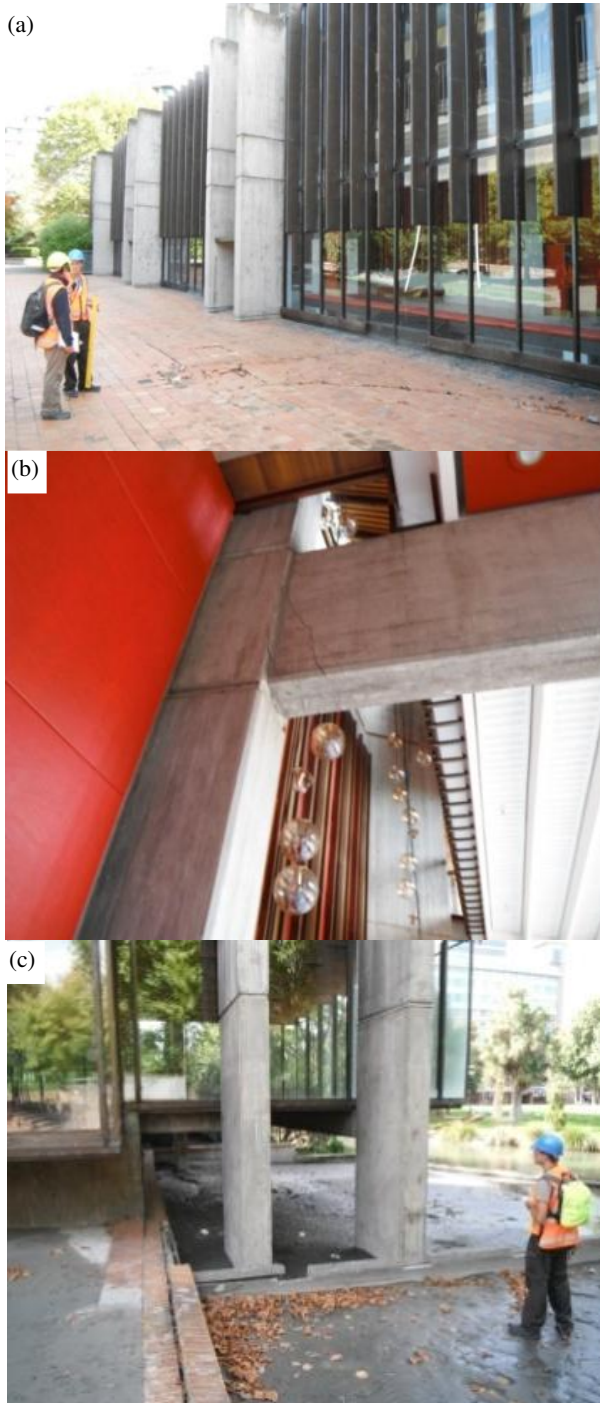
Figure 14: Town Hall auditorium and adjacent dining facility undergoing significant liquefaction-induced differential settlement and lateral movements [7].
