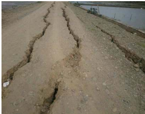
Fig. 11. Ground failure in Manohara-shorelines Pidie Jaya Aceh earthquake 7th December 2016.
