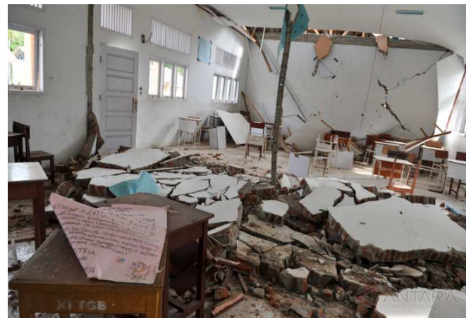
Fig. 9 Failures of school due to high amplification of seismic ground motion inducing foundation failure.
