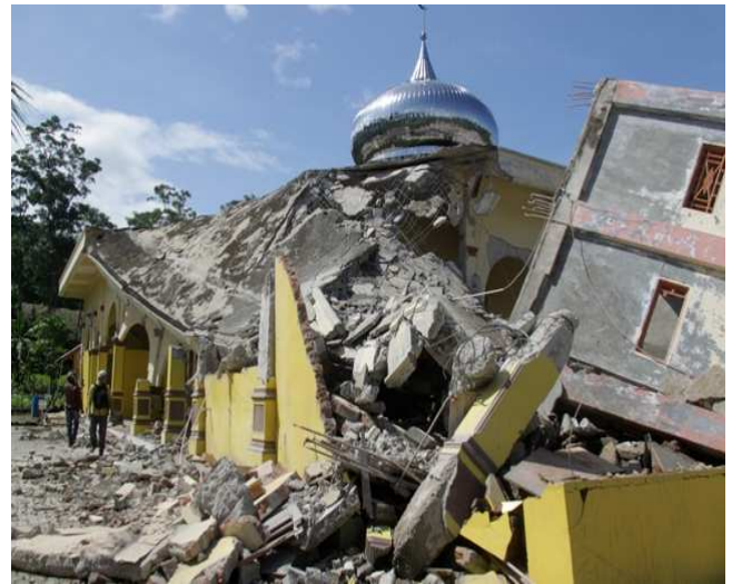
Fig. 8 Failures of vulnerable mosque due to high amplification of seismic ground motion inducing foundation failure.
