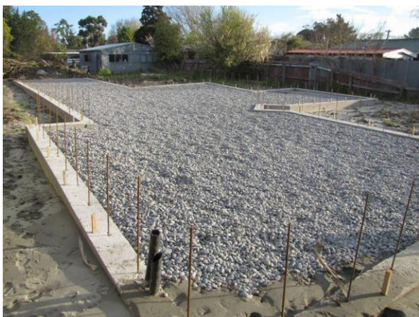
Figure 5.41: Site at Pines Beach which appears to be using the same slab-on-grade system as at Bexley (Chichester Street)
