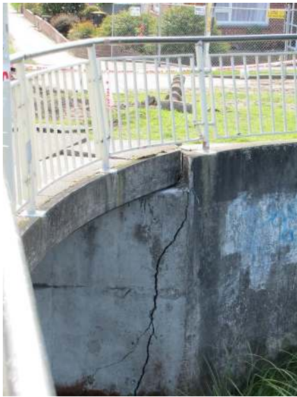
Figure 7.14: Cracking of north abutment, Swanns Road Bridge.
