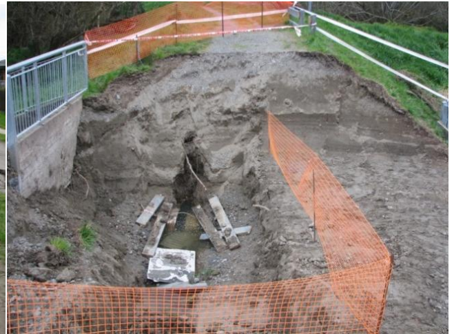
Figure 6.26: Photo 28: Failed drainage conduits running underneath the stopbank on the south side of the Kaiapoi River. The location of this photograph is denoted in Figure 6.2. (43.388679°S, 172.666203°E).
