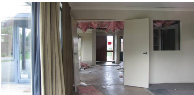
Figure 5.45: Interior view of residence at Riverside Lane. Note the two floor breaks visible in the picture
