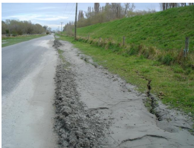
Figure 6.5: Photo 2: Crack running along base of stopbank on Coutts Island Rd (landside) and liquefaction ejecta. (43.424466°S, 172.629907°E).
