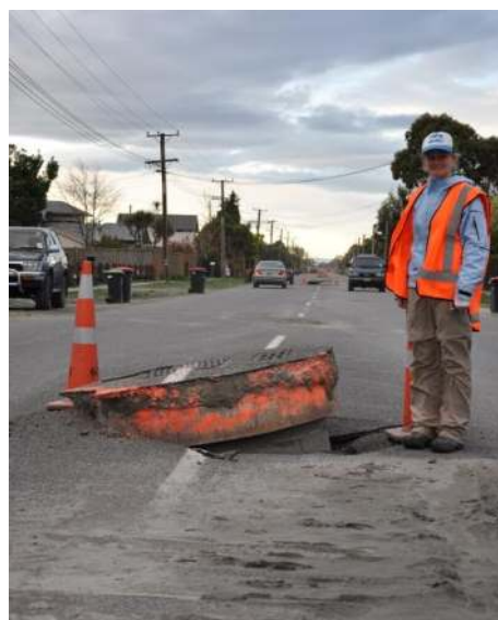
Figure 7.47: Uplifted manholes along Lower Styx Road, note the continuation of pattern in the foreground (43.4113°S, 172.6930°E).
