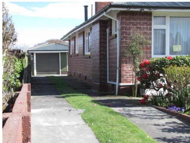
Figure 5.26: Residence affected by lateral spreading along the driveway which has induced differential settlement between the front and rear of the house. (Note that this is not a slab-on-ground house, rather an older style of construction with a concrete perimeter beam and the timber floor being supported on shallow foundations; Locksley Ave).
