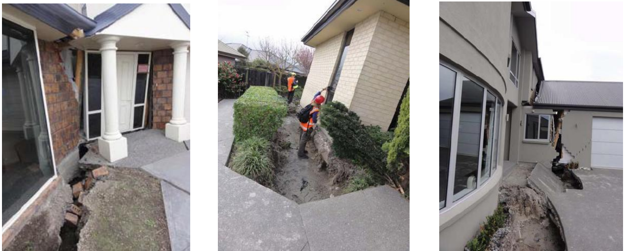
(b) Effects of lateral spreading in residential area.
