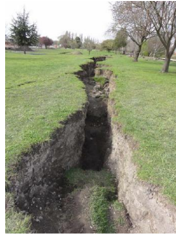
(b) Lateral spreading of the north stopbank of Kaiapoi River (Charles St – Jones St).
