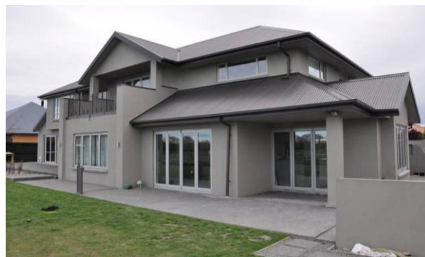
Figure 5.23: Damage to a residence along Courtenay Drive in the South Kaiapoi residential community. Rear of home facing Paddocks field articulates relatively no damage.
