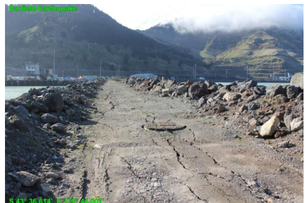
Figure 7.39: Cracking along jetty at eastern end of port.
