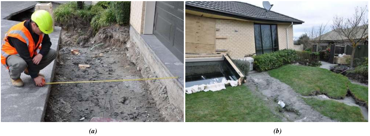
Figure 5.22: Damage to a residence at Courtenay Drive in the South Kaiapoi residential community (a) front of home (1.5 m separation between garage and approach slab) and (b) back of home.
