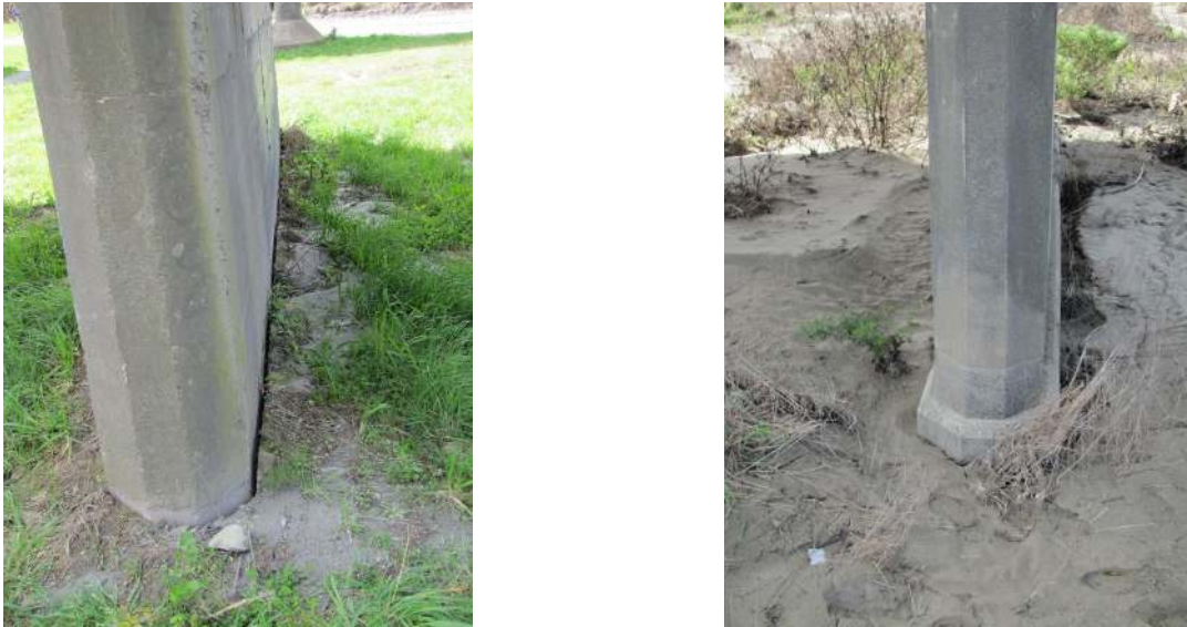
Figure 7.29: Evidence of liquefaction at Highway 1 bridge piers on the north side of the Waimakariri River.
