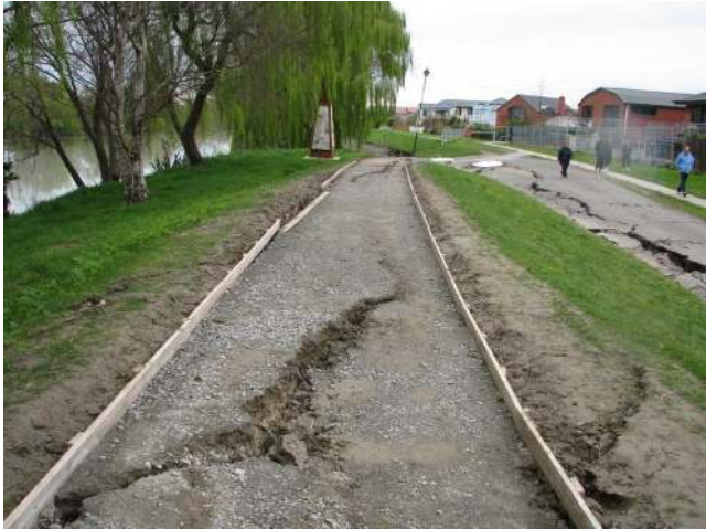
Figure 6.25: Photo 27: Lateral spread cracks along the top of the stopbank on the south side of the Kaiapoi River. The location of this photograph is denoted in Figure 6.2. (43.385693°S, 172.660688°E).
