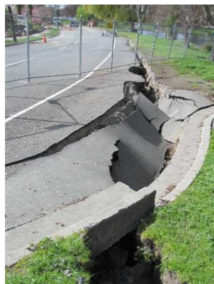
Figure 7.11: Lateral spreading on west approach fill, Swanns Road Bridge.
