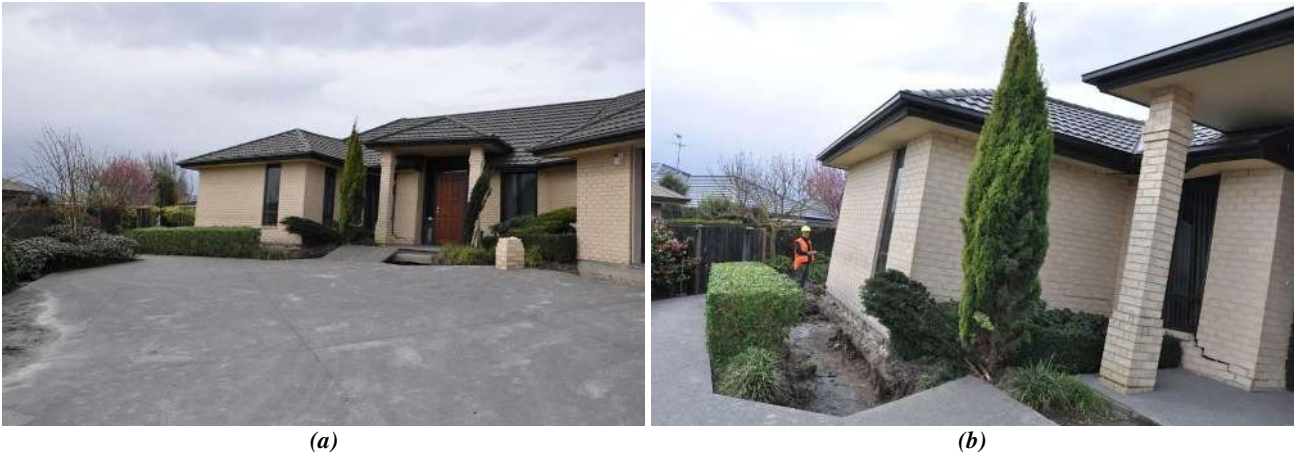
Figure 5.21: Damage to a residence at Courtenay Drive in the South Kaiapoi residential community (front of home articulating excessive tilt and separation of foundation from surrounding hardscape).
