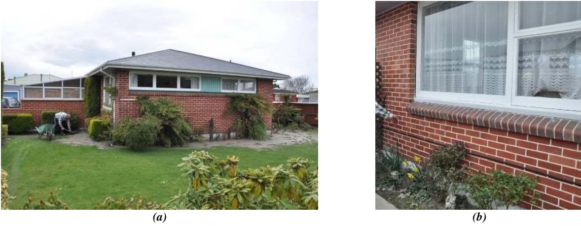
Figure 5.15: Residence along Charles Street. (a) Ejecta surrounding home and (b) owner points out shear cracking and gapping developed between window and brick due to structures movement.
