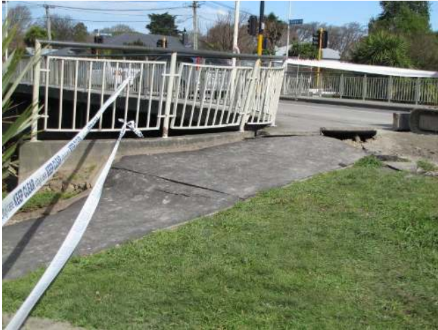
Figure 7.12: Incipient lateral spreading at west abutment, Swanns Road Bridge.
