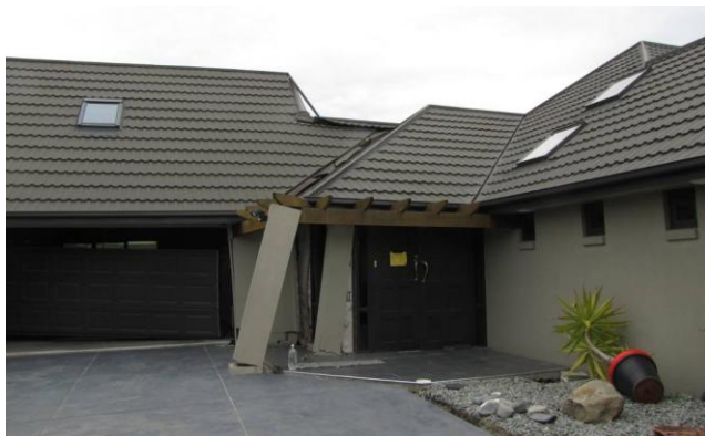
Figure 5.47: House with fissured floor slab with damage carried through to the roof line which is no longer weather proof. (Riverside Lane, Spencerville).
