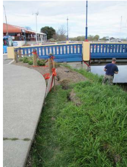
Figure 7.18: Incipient lateral spreading of east abutment, Williams Road Bridge.
