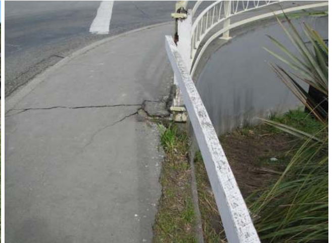
Figure 7.13: Incipient lateral spreading at north abutment, Gayhurst Road Bridge.
