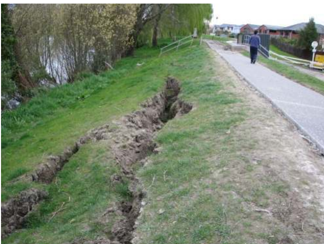
Figure 6.23: Photo 25: Lateral spread cracks along riverside stopbank on the south side of the Kaiapoi River. The location of this photograph is denoted in Figure 6.2. (43.385254°S, 172.660131°E).
