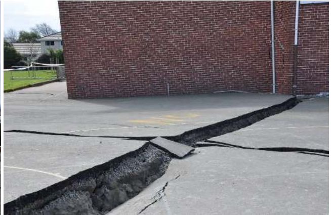
Figure 5.31: St. Paul's church in Dallington area - view looking north at ground failure, which continued through the building.
