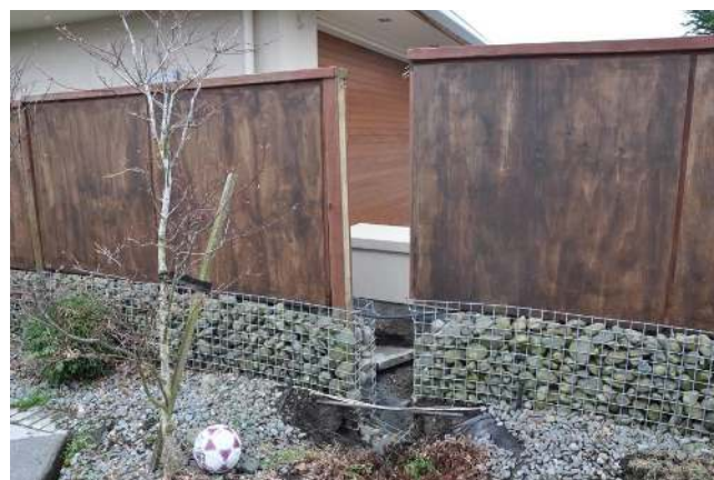
Figure 5.48: Separated fence line due to propagating ground fissure meandering between homes along Riverside Lane.
