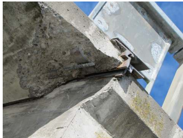
(a) West abutment gap closure and spalling.
