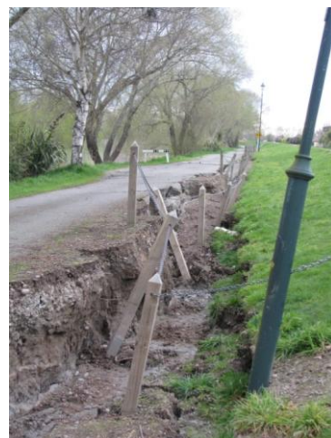
Figure 6.24: Photo 26: Lateral spread cracks along the riverside stopbank on the south side of the Kaiapoi River. The location of this photograph is denoted in Figure 6.2. (43.385839°S, 172.660941°E).
