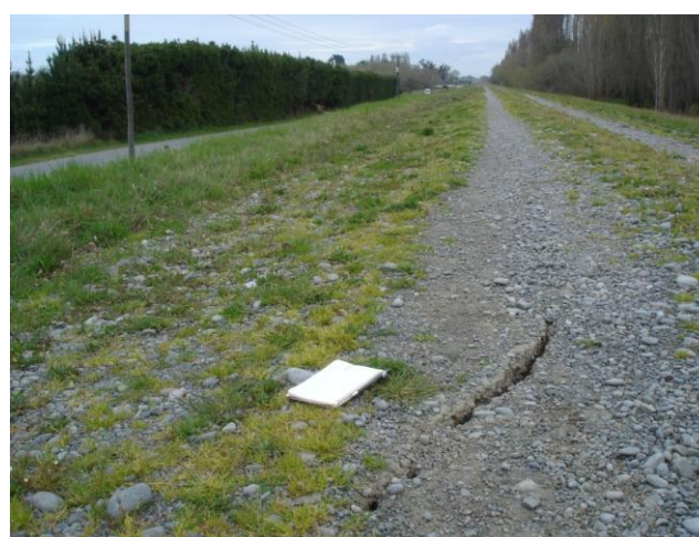
Figure 6.8: Photo 5: ~20 mm wide crack running lengthwise along the top of the stopbank on Coutts Island Rd. This crack was at the edge of the ~0.5 km stretch of the stopbank where significant liquefaction was observed. Photo taken looking southwest (43.423440°S, 172.632349°E).
