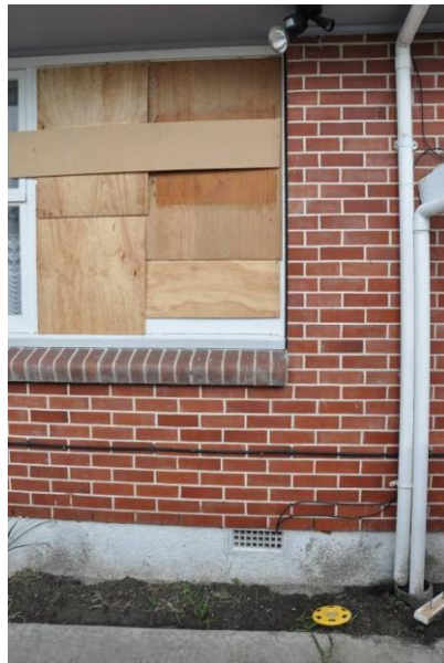
Figure 5.16: Residence along Charles Street (same structure as Figure 5.16). Damage to glass windows and between window and wall.
