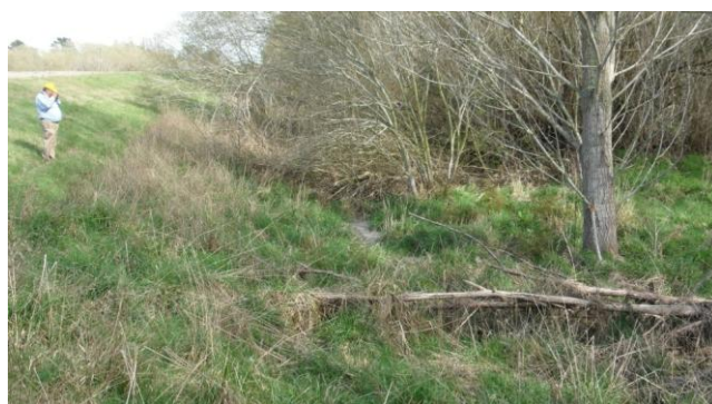
Figure 6.6: Photo 3: Liquefaction ejecta (centre of photo) along the base of the stopbank on Coutts Island Rd (riverside). (43.424093°S, 172.630468°E).
