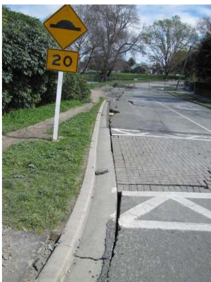
Figure 7.10: Cracking of roadway on west approach fill, Swanns Road Bridge.
