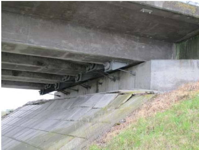
Figure 7.22: Cable Restrainers at north abutment, Chaney's Overpass.
