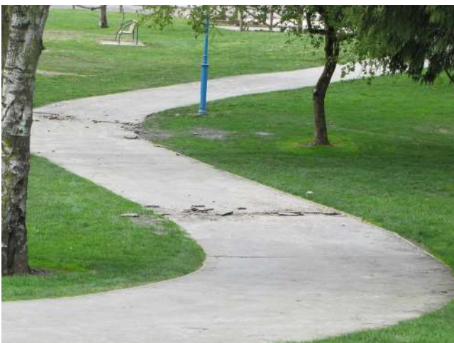
Figure 7.20: Cracking of sidewalk and evidence of liquefaction in Trousselot Park.
