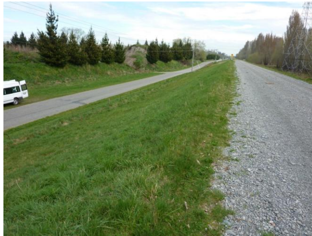
Figure 6.9: Photo 6: Stretch of stopbank without evidence of liquefaction. In the distance, a small rise can be seen in the road. This rise is the start of the ~0.5 km stretch where liquefaction was observed along the base of the stopbank. (43.4225°S, 172.6350°E).
