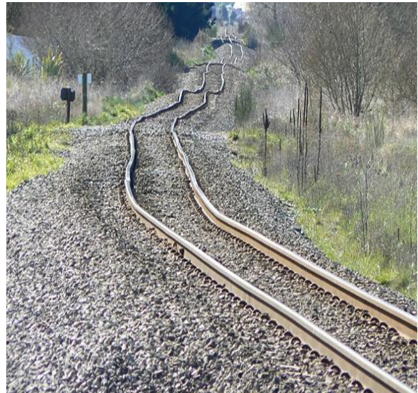
Figure 7.36: Damage to rail line at Woodford Glen (photo by L. Matthews and J. Overend).
