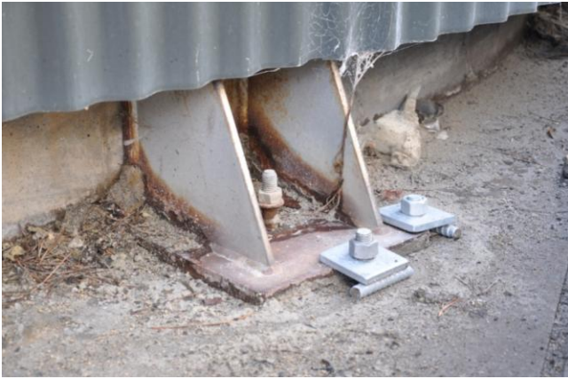
Figure 7.43: Typical repair to Tank 3 and 4 (addition of clamp plates). Note the pullout of the original anchorage. Fulton Hogan Bitumen Plant. (43.6085°S, 172.7149°E).
