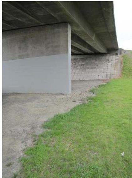
Figure 7.24: Evidence of liquefaction beneath Chaney's Overpass.
