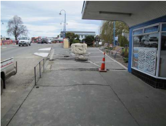
Figure 7.17: Cracking of east approach roadway, Williams Road Bridge.
