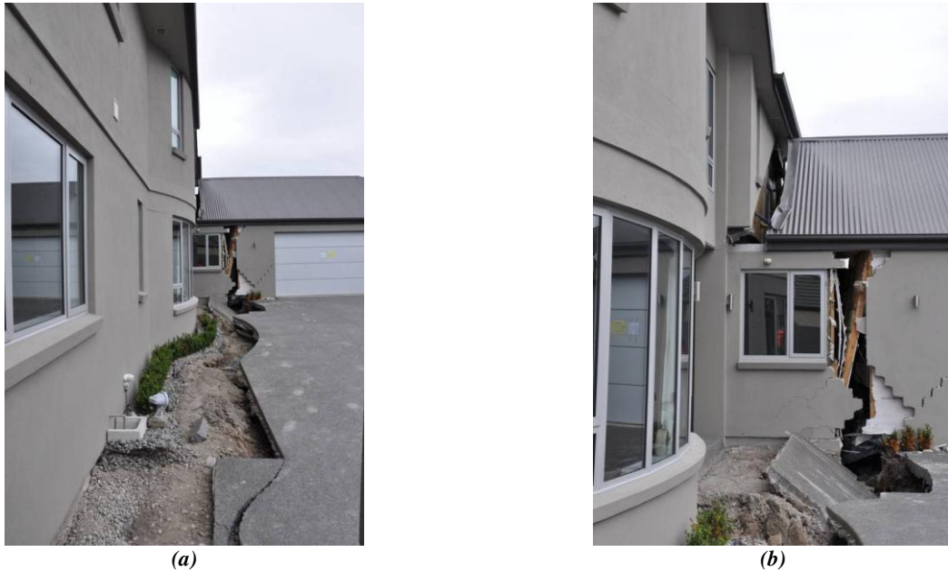
Figure 5.24: Damage to a residence along Courtenay Drive in the South Kaipoi residential community. Front entry articulates extensive damage as large ground spreading subtends into the superstructure.
