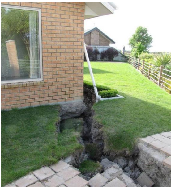
Figure 5.38: Lateral spreading compromising ground support beneath the concrete slab-on-grade house foundation. (Kokopu Street).
