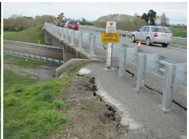
Figure 7.21: Incipient lateral spreading at Chaney's Overpass north abutment.
