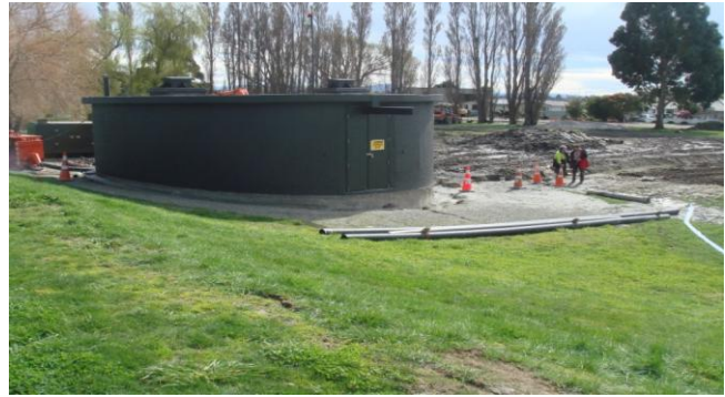
Figure 6.21: Photo 22: Settlement of tank structure. The locations of these photographs are denoted in Figure 6.2. (43.386918°S, 172.664412°E).
