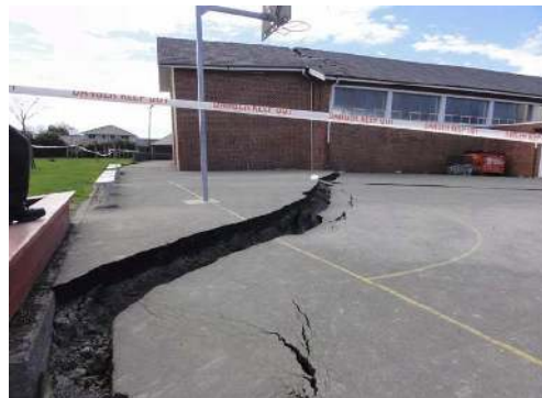
(a) Bearing failure in liquefied soils (St Paul's Church, Dallington); the crack is 500-900 mm wide with a vertical offset of 330 mm, at its maximum.
