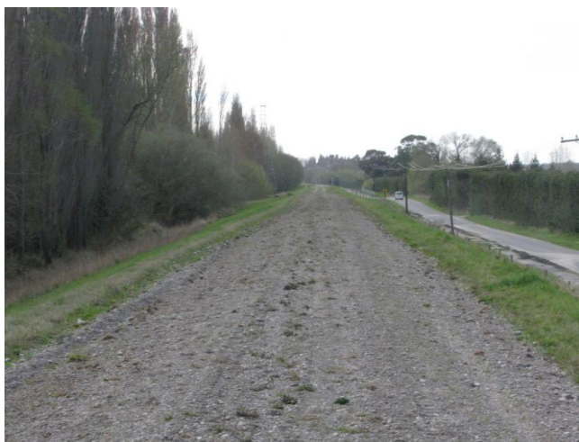
Figure 6.7: Photo 4: Road on top of stopbank that had recently been regraded, presumably after the earthquake to fill in longitudinal cracks formed during the earthquake. Liquefaction was observed along the base of both sides of the stopbank along this stretch. (43.423943°S, 172.631045°E).
