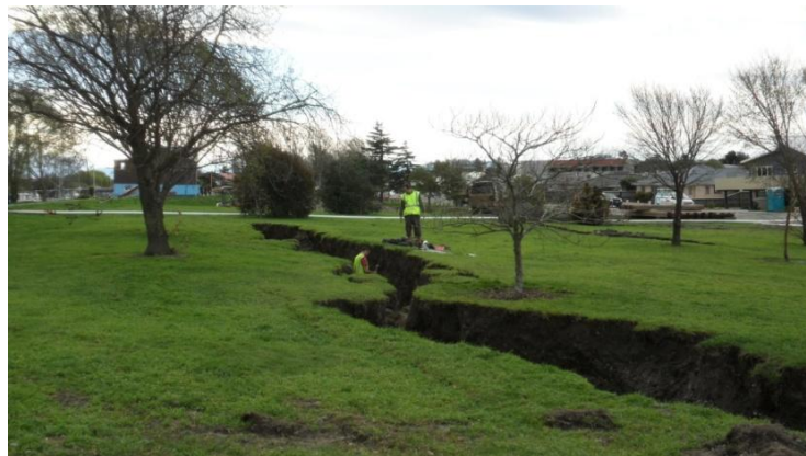
Figure 6.18: Photos 16-18: Lateral spread cracks along landside of the stopbank on the north side of the Kaiapoi River. The locations of these photographs are denoted in Figure 6.2. (43.384484°S, 172.660653°E).
