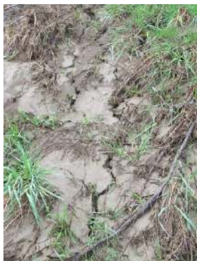
Figure 4.37: Ground damage adjacent to the bank of the Selwyn tributary near the end of Gillanders Rd (Darfield side). (Position marked as Photo 1 in Fig. 4.36).
