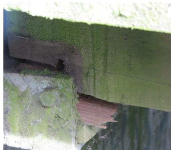
(b) Sheared bearing on east bank.
