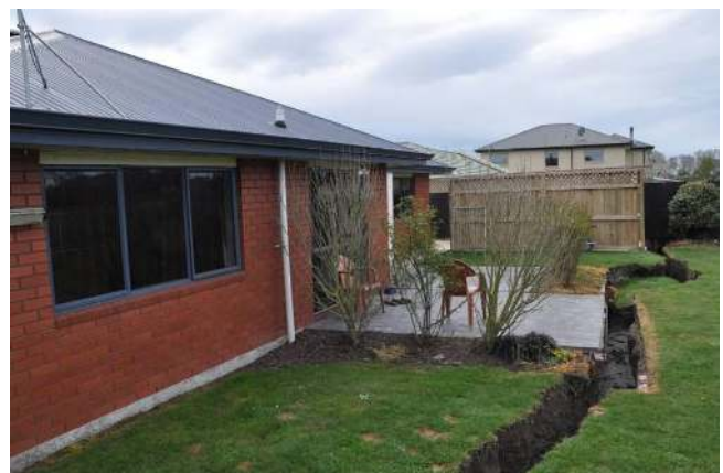
Figure 5.20: Ground failure feature extending through the backyard of a home on the south side of Courtenay Drive in the South Kaiapoi residential community.
