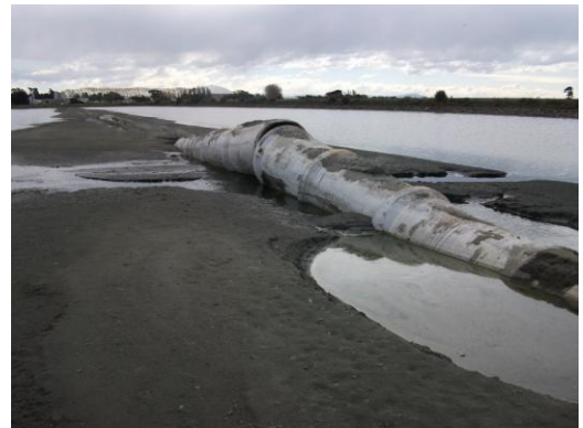
Figure 6.32: Buckled pipe protruding from Pond 1 during pond dewatering, and after pond level was lowered. Pipeline crown was at the pond invert prior to the earthquake. (-43.530867°, 172.705190°).
