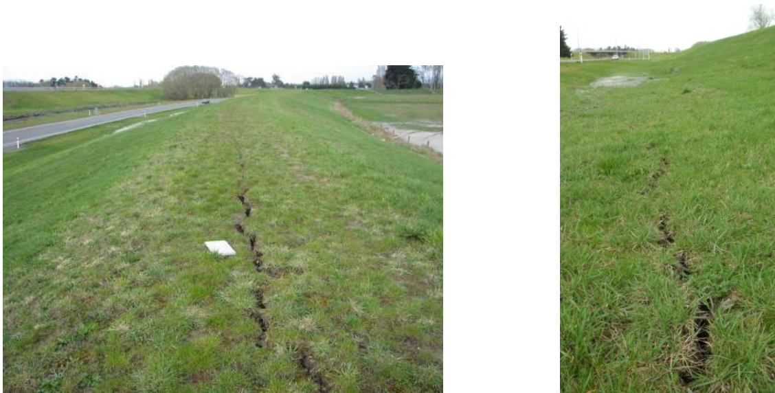
Figure 6.15: Photos 9 and 10: ~50 mm wide longitudinal cracks running along the crest (left) and base (right) of a secondary stopbank for the Waimakariri River. Photo taken looking southwest; SH1 on left of stopbank (43.430108°S, 172.643434°E).
