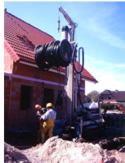
Photo 1. Installation of borehole heat exchanger at a small house in Bielefeld, Germany, using a small, powerful Rotomax drilling rig.
