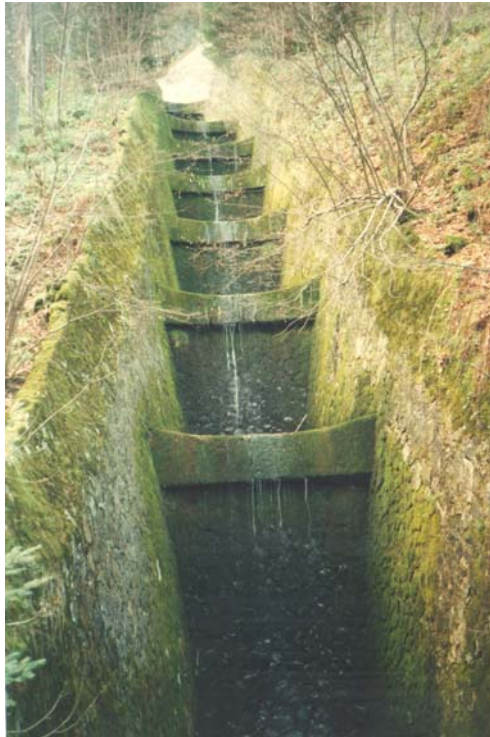
(b) View from downstream of the masonry stepped spillway located on the left bank.
