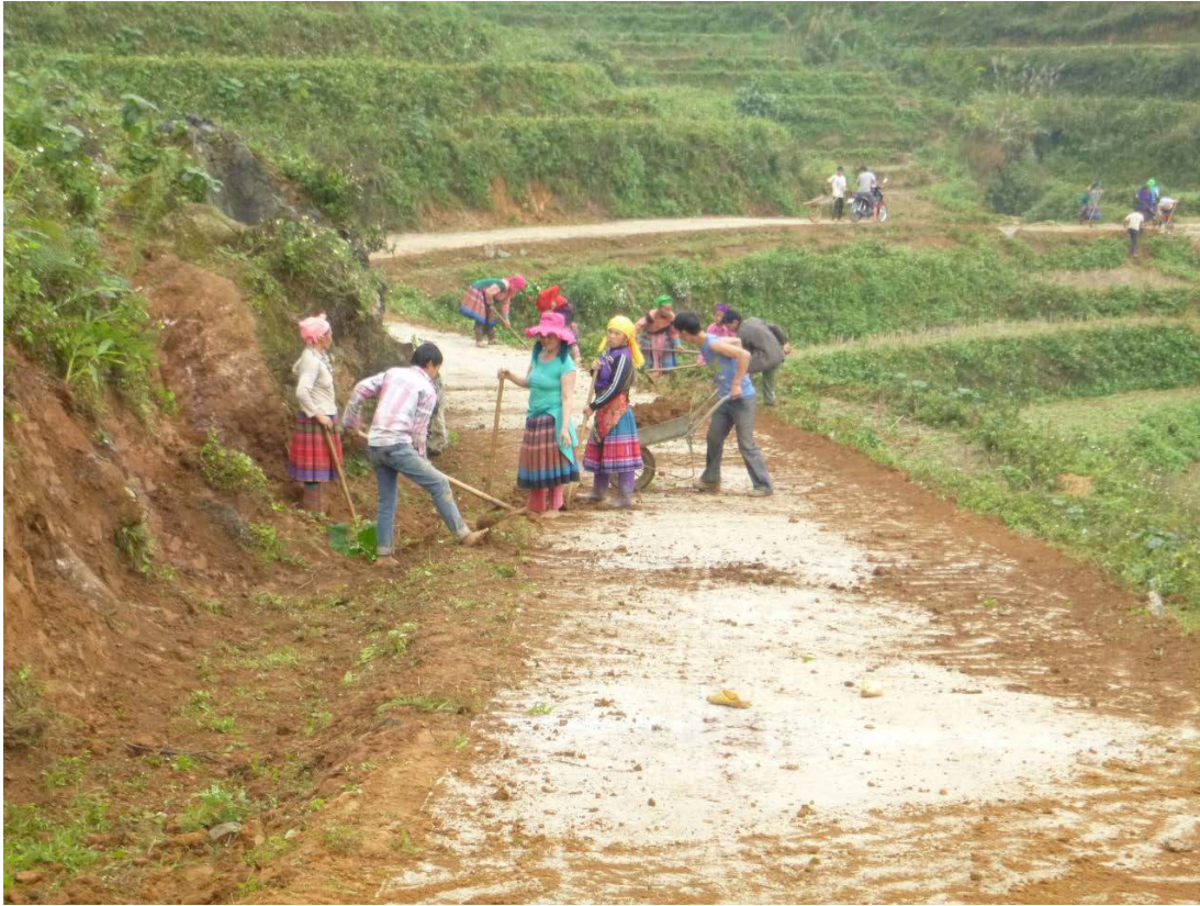
Photo 5.2: Villagers working on a rehabilitated commune road under the ‘New Rural’ programme of the government
