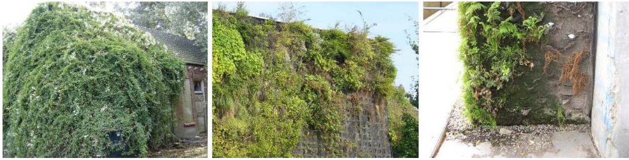
Figure 3. Examples of possible damages due to the lack of maintenance and to design mistakes.
