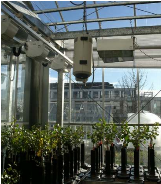
Fig. 3 An aspirated sensor box suspended centrally in free air for recording environmental parameters. The sensors are located inside the box while air is constantly drawn through the box. Sensor (box) type and location along with frequency of sampling and details of data integration should be reported.
