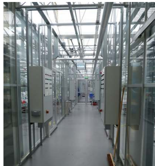
Fig. 4 Greenhouse environmental control systems are diverse and frequently control algorithms are specific to the particular size, structure, orientation and location of the facility. Pertinent information on the system should be reported.
