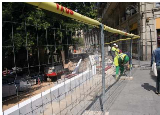
Figure 13. Laborers working on the construction of a “podium” to enhance the Roman Walls of Barcelona, street Tapineria, on May 2016. Ana Pastor.
