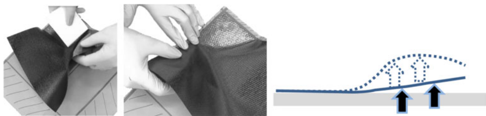
Figure 12 Example of folding material to accommodate the shear during task 8 (not to scale)
