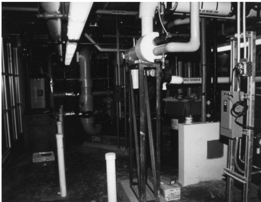
Fig. 6. Exposed features of the building demonstrate how buildings function. In this case, the mechanical room is exposed, with color-coded piping.
