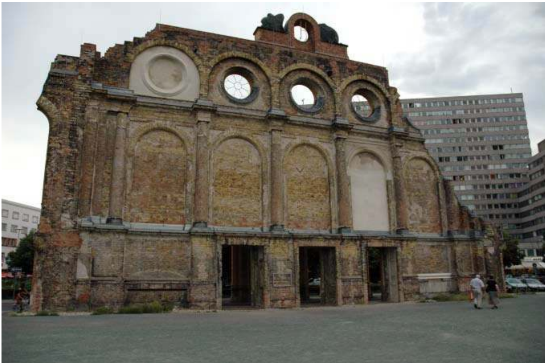
FIGURE 4. Façade of the Anhalter Bahnhof, Berlin, showing patching. Photograph by the author, June 2007.
