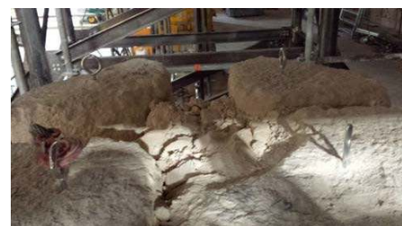
Figure 8. Top images of a pillar during disassembly; in the centre, the irregular mortar core of the column
