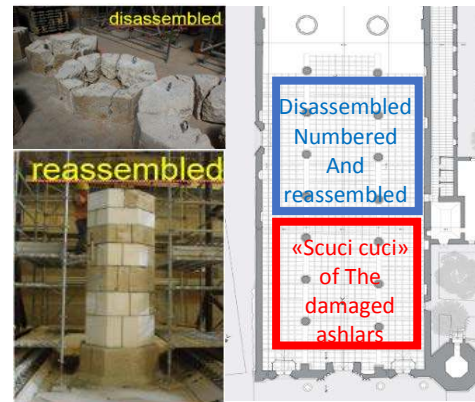
Figure 11. The two different conservation activities planned on the pillars in the design project: global disassembly & reassembly of the stone ashlars with approximately 50% of the stone volume saved and 50% replaced (red); «scuci cuci» proposal with punctual replacement of the single damaged stone ashlars (blue)
