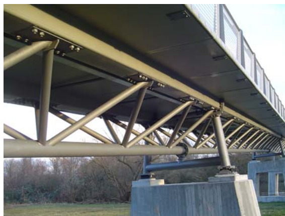
Fig. 1 Gärtnerplatzbridge in Kassel, Germany (2007), consisting of a high performance deck glued to a 3-D steel truss
