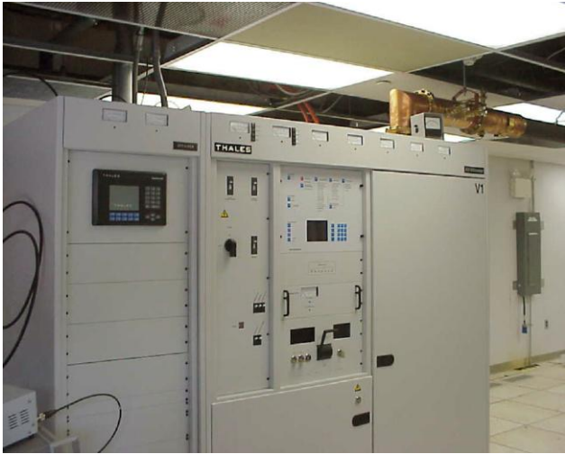
Fig. 9 SRF 50 kW transmitter
