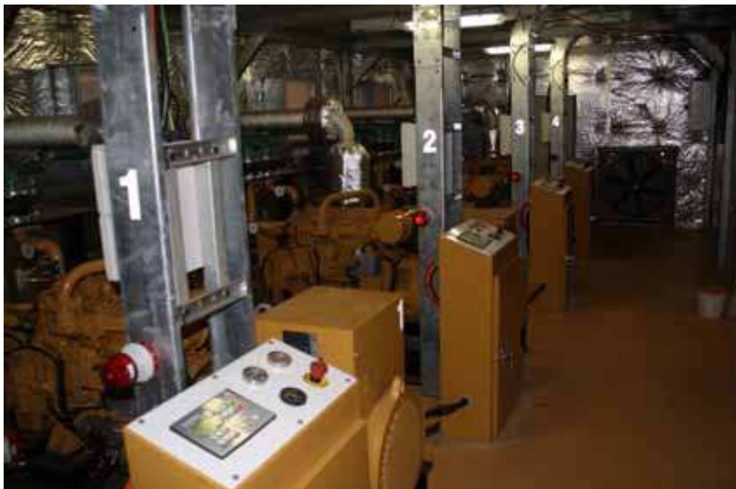
Fig. 19. Diesel Room at Eco Beach Resort
