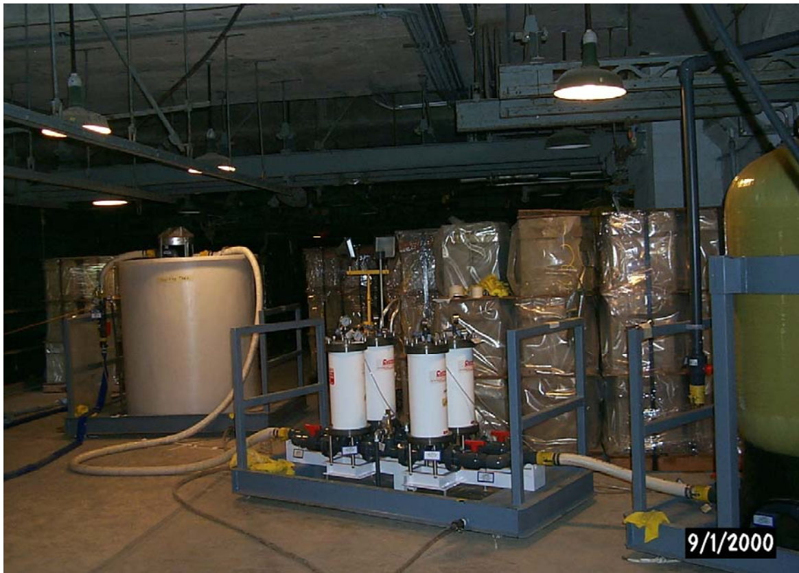
Fig. 1; Graver/Selion System in R-Basin: Activated Carbon Tank to the Right, with the 1 and 5 Micron Filters in the Center, and the CsTreat® Inside the Shielding Tank to the Left
