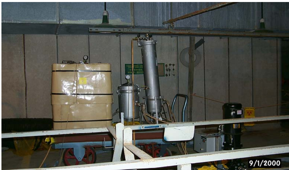
Fig. 2 – 3M Cs-137 Removal System in the R-Reactor Disassembly Basin. The 4-foot tall, 6-inch diameter, 2-micron pre-filter is to the right and a small tank with nine 0.2-micron pre-filters is in the center. The 22 SSC™ Cs-137 removal filters are inside a stainless steel tank to the left, which was covered with ~1 inch of lead shielding to reduce the gamma dose.
