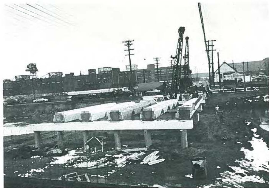
Fig. 24. Post-tensioned box girders on which pretensioned slab sections were placed. Topping was cast over the top of the deck section to provide a composite deck with girders and pretensioned slab sections.
