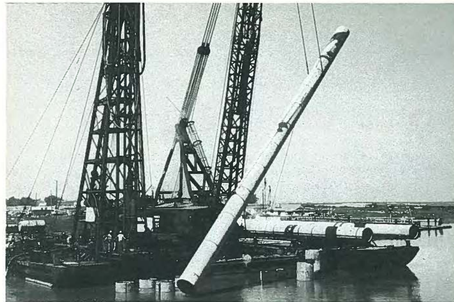
Fig. 52. Napa River Bridge, California: pretensioned monolithic cylindrical pile, 54 in. diameter, 120 ft long. It is believed to be the first such pile used worldwide.
