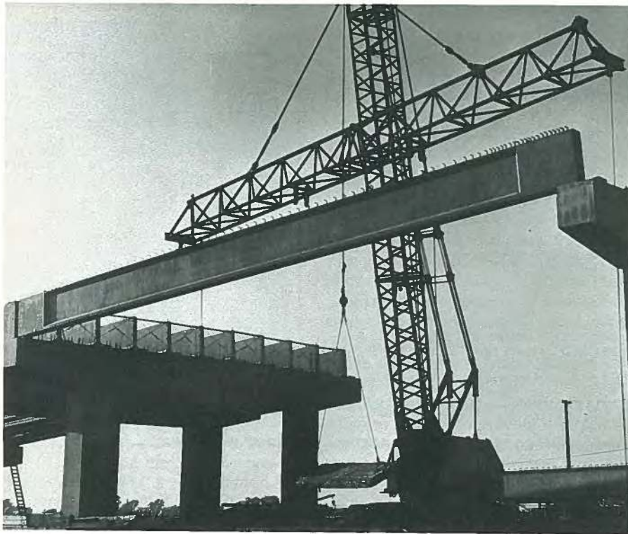
Fig. 49. Napa River Bridge, 1957: one of the earliest applications of prestressed deflected strands. Design by California State Department of Highways.
