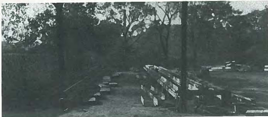
Fig. 16. Fabricating beds at a Breeko plant for producing prestensioned channel slabs with deflected strands. Built in March 1953.
