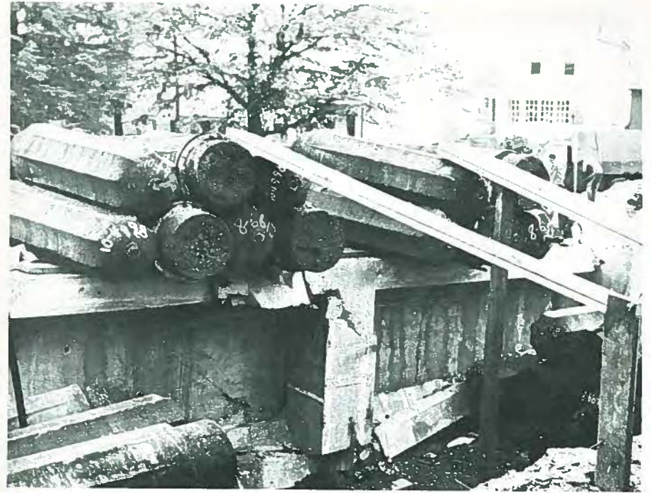
Fig. 18a. Closeup of failure at midspan.
