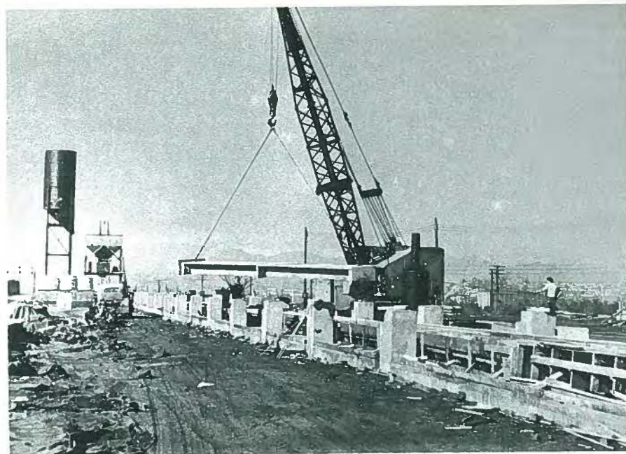
Fig. 11. A single-tee slab is lifted off the bed ready for transport to the Spitzer Electric Company.
