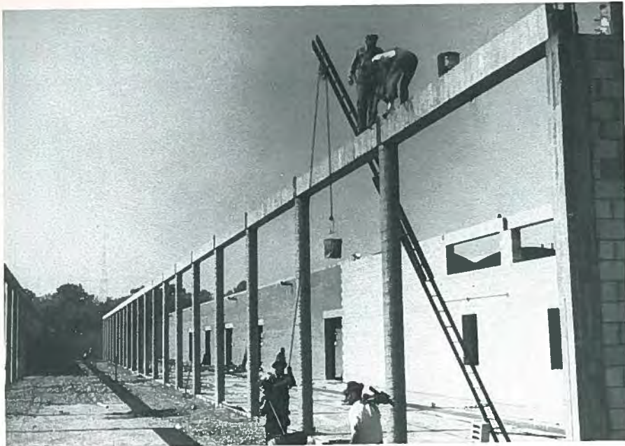
Fig. 12. Grouting continuity steel in 12 x 16-in. (305 x 406 mm) block beams of 40,000 sq ft (3720 m 2 ) warehouse for General Shoe Corporation.
