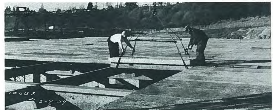
Fig. 65. Lightweight roof slabs are lowered, two at a time, into place across the structural frame. The precast slabs are 40 in. (1.02 m) wide, 10 ft (3.05 m) long and 1½ in. (38.1 mm) thick, with a 6-in. (152 mm) leg.
