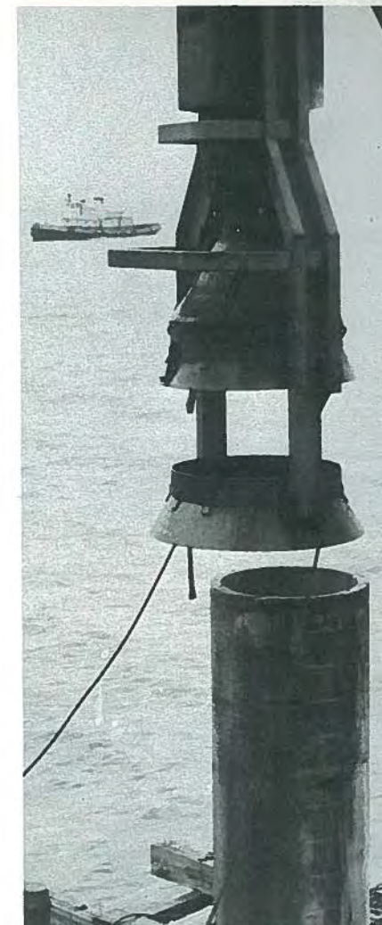
Fig. 3. Close-up of the driving of a 96-ft long 54-in. diameter cylindrical pile in 1953 for the Lake Pontchartrain Causeway. Note special driving bonnet which had to be engineered.
