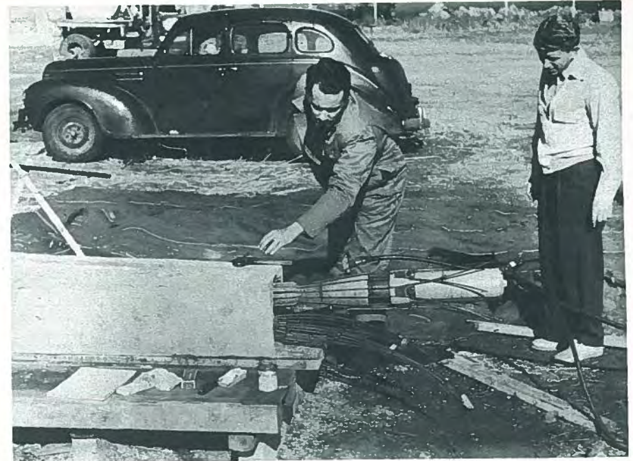
Fig. 28. Jean Muller (left) and Jack Perlmutter work together on the post-tensioning of a beam to be used with pretensioned channel slabs for Denver Livestock Feed.
