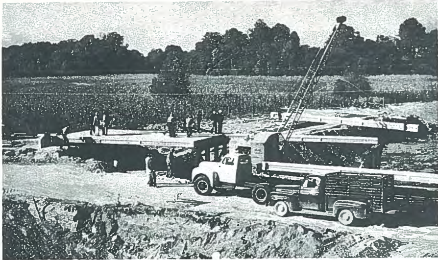
Fig. 10a. Erection of block-beams hauled 176 miles from fabricating plant to erection site, Obion County, Tennessee (about 1950).
