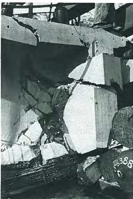
Fig. 12. Closeup of fracture zone of Walnut Lane test girder. Failure was in the top flange to right of the stiffener.
