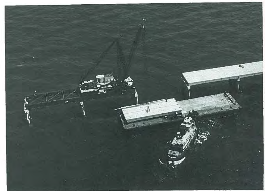
Fig. 7. General view of erection of a span to be part of the Chesapeake Bridge-Tunnel Crossing connecting Cape Charles to Norfolk, Virginia.
