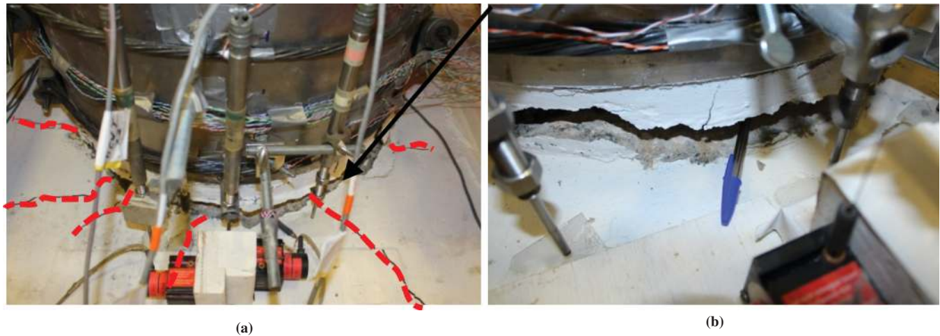
FIGURE 8 Concrete cracks associated with stress transfer through dowel bars at the column-footing connection: (a) cracks on footing and (b) damage in the plastic hinge (footing cracks marked with red dashed lines).
