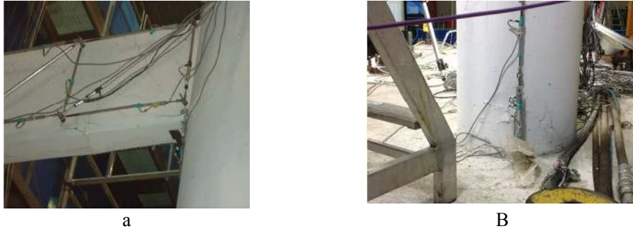
Figure 19. Close-up views of Pier #11: a) transverse beam; and b) left column, after HS k09.
