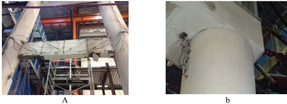
Figure 23. Damage state of Pier #11 after HS k12: a) transverse beam damage; b) crack opening underneath the cap beam.
