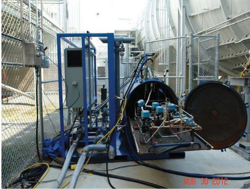
Figure 15. One of the two portable valve pallets with sealed tank open at the outside test stand. The intrinsically safe control cabinet is shown on the left.
